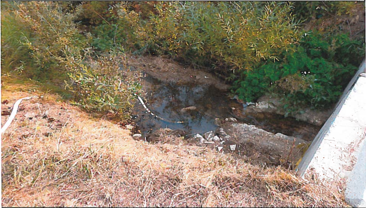
Point of Diversion: View of 1 1/4" suction line in Pyle Creek. A concrete dam, shown at the right, with boards, creates a pool upstream in which to pump water for irrigation.
