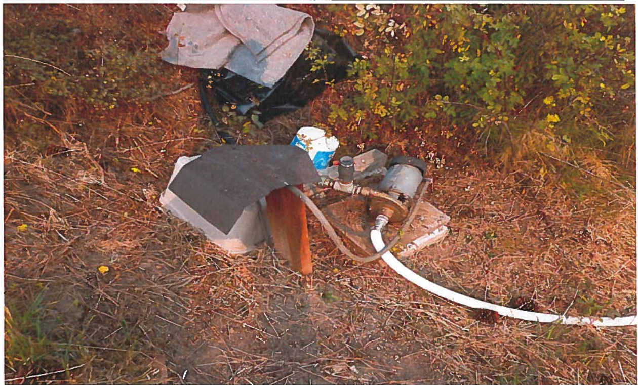
View of 2 hp pump and 1 1/4" suction line from Pyle Creek. Pump is located at top of bank adjacent to Pyle Creek.
