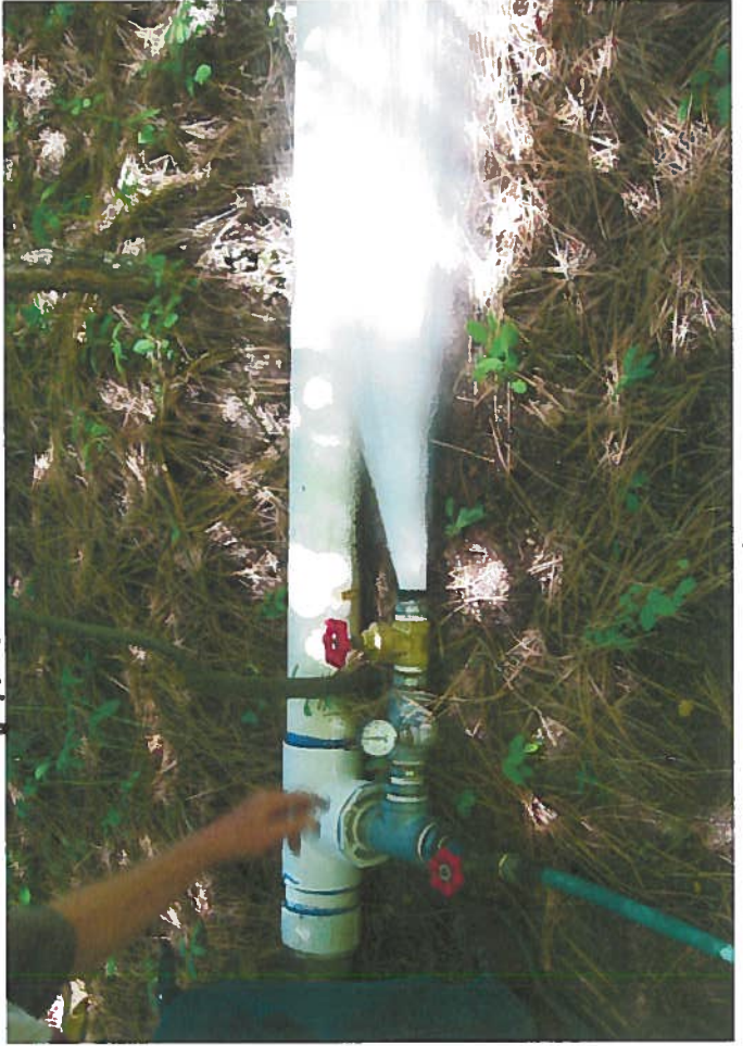
FIRE PORT / IRRIGATION PORT.
