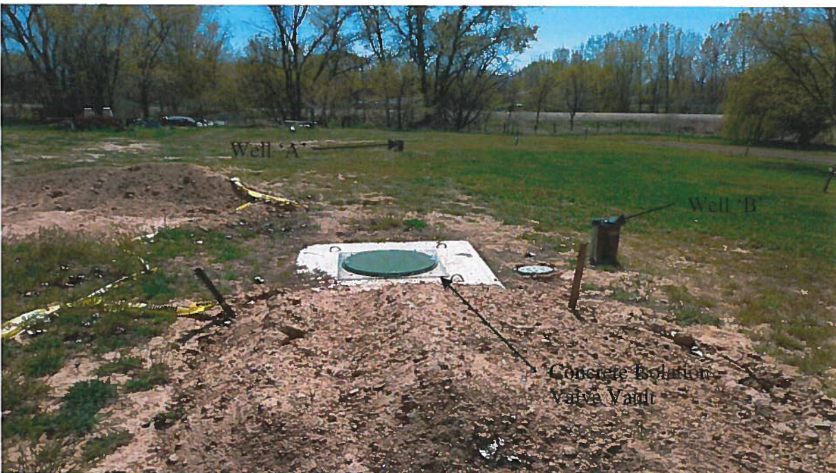
Point of Diversion: View southwesterly of Well 'A' and Well 'B'. The concrete vault near Well 'B' contains the isolation valves to each 3" discharge line from the wells. The two 3" well discharge lines are connected to form one 3" main discharge line to the three pressure tanks in the mechanical room of the office building.
