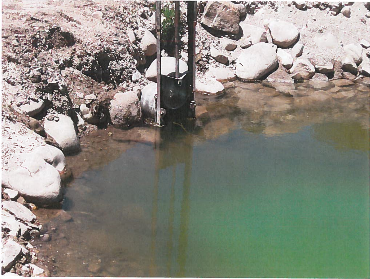
Control structure on outflow pipe
