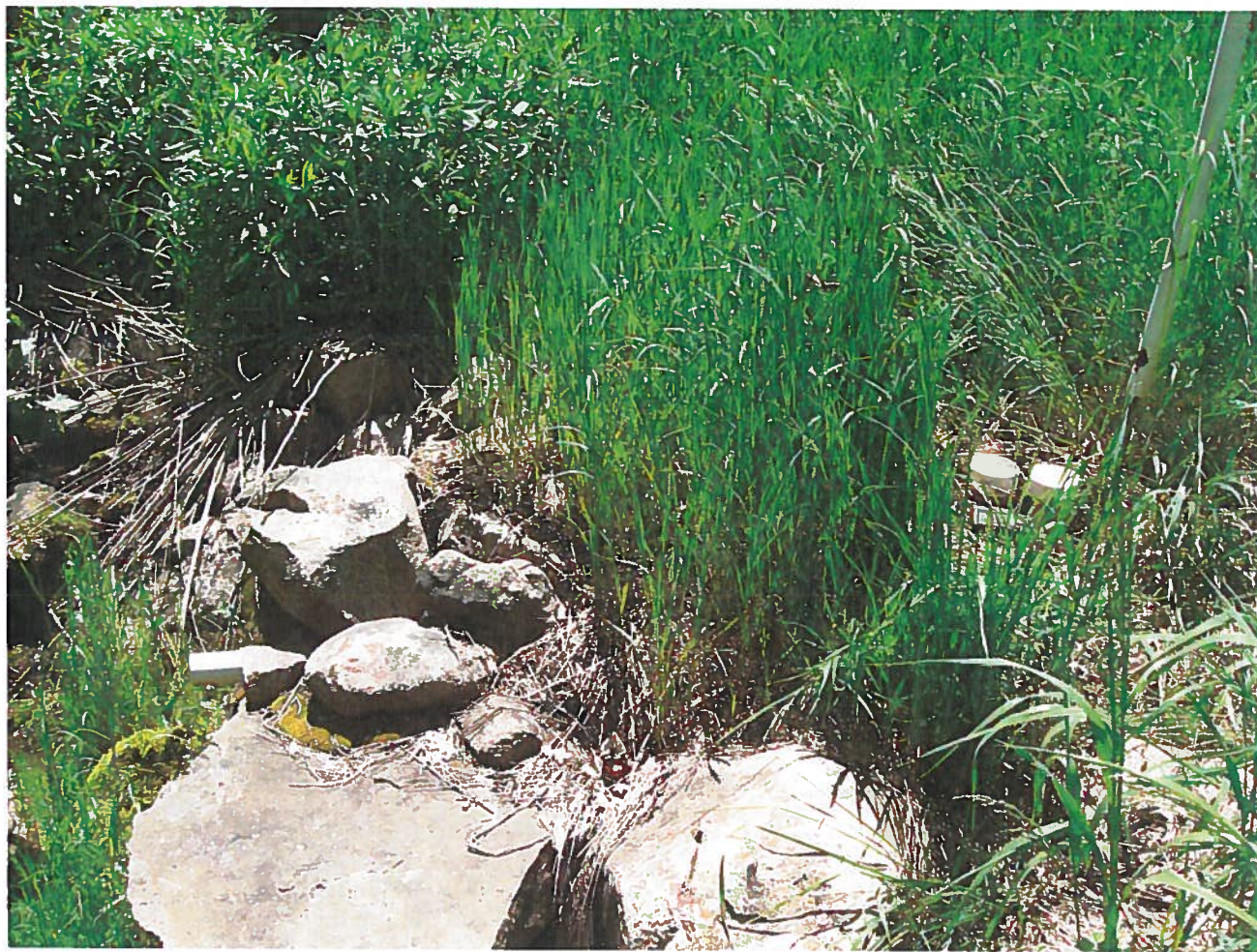
Spring box and overflow pipe
