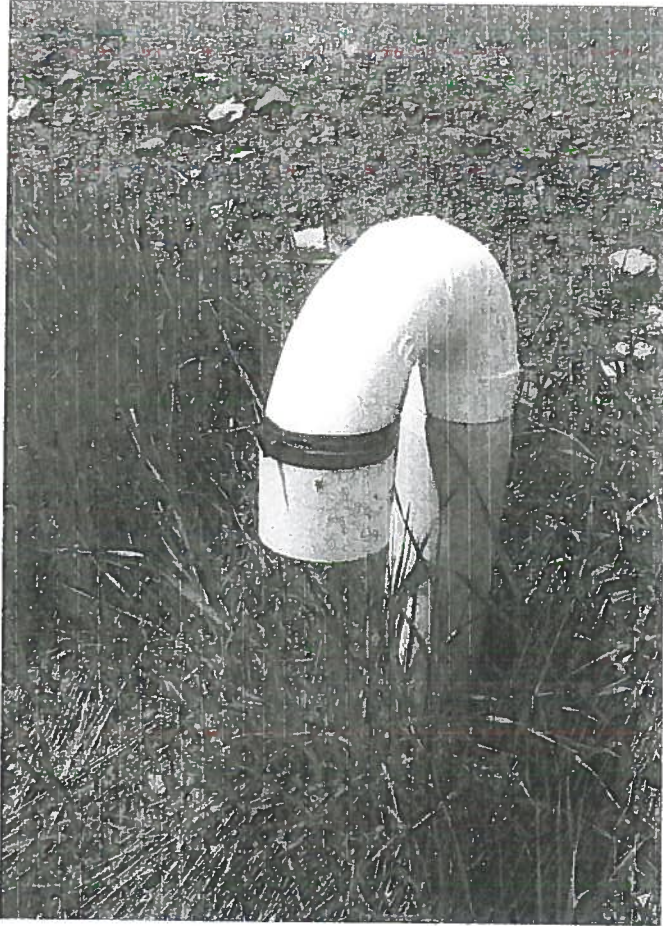
Photo #6 Storage Tank Overflow
