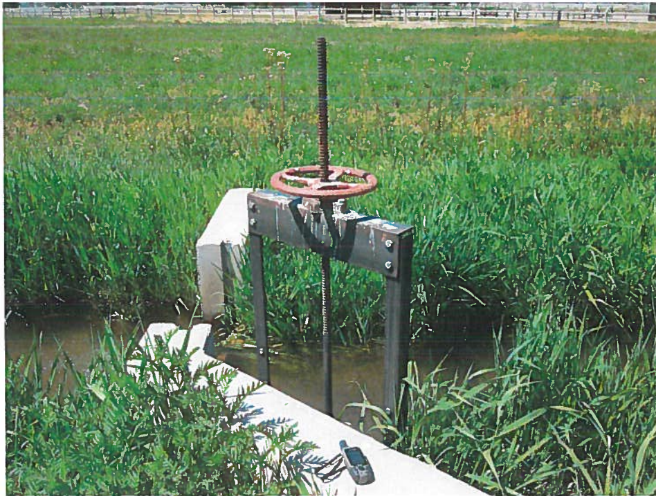
Figure 4: Headgate on Lateral to Ditch
