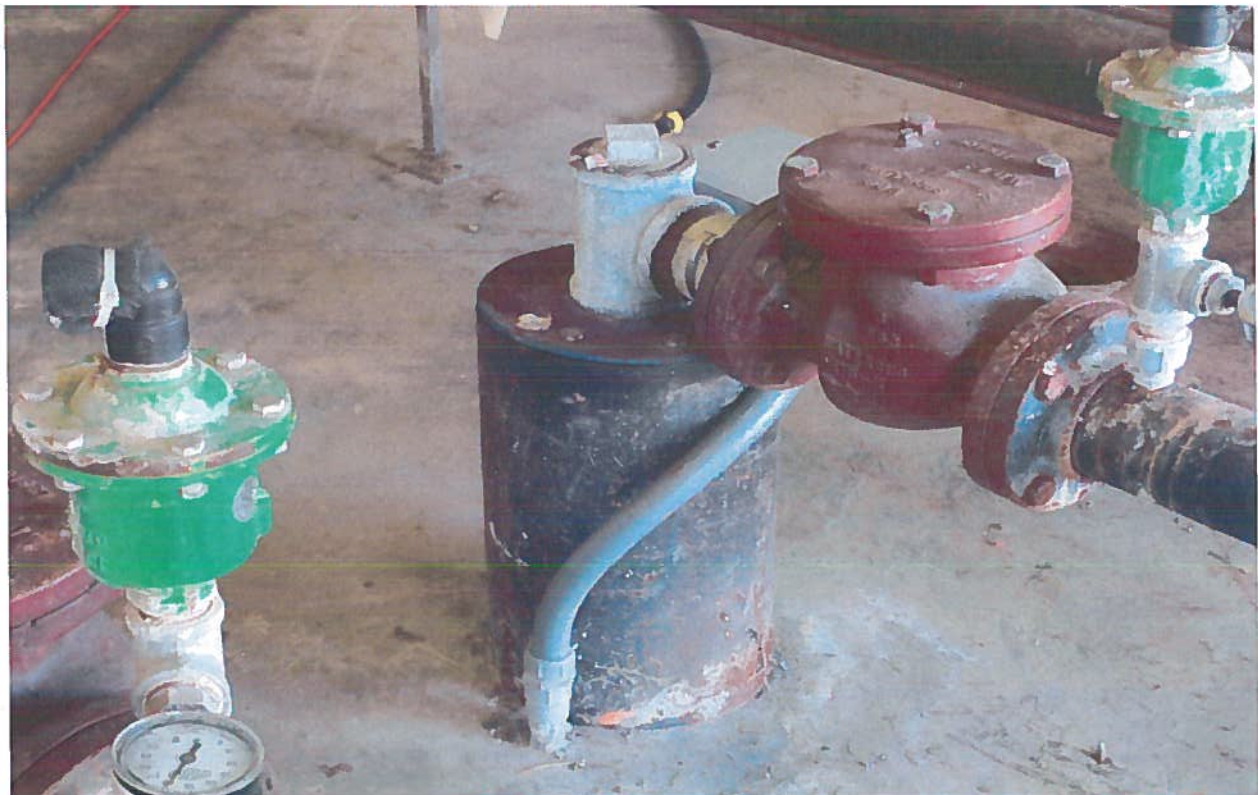
West well inside wellhouse
