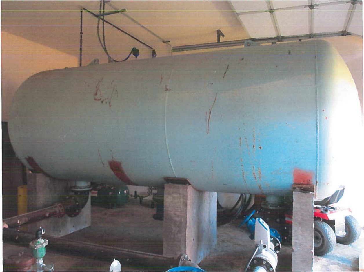
Pressure tank in wellhouse
