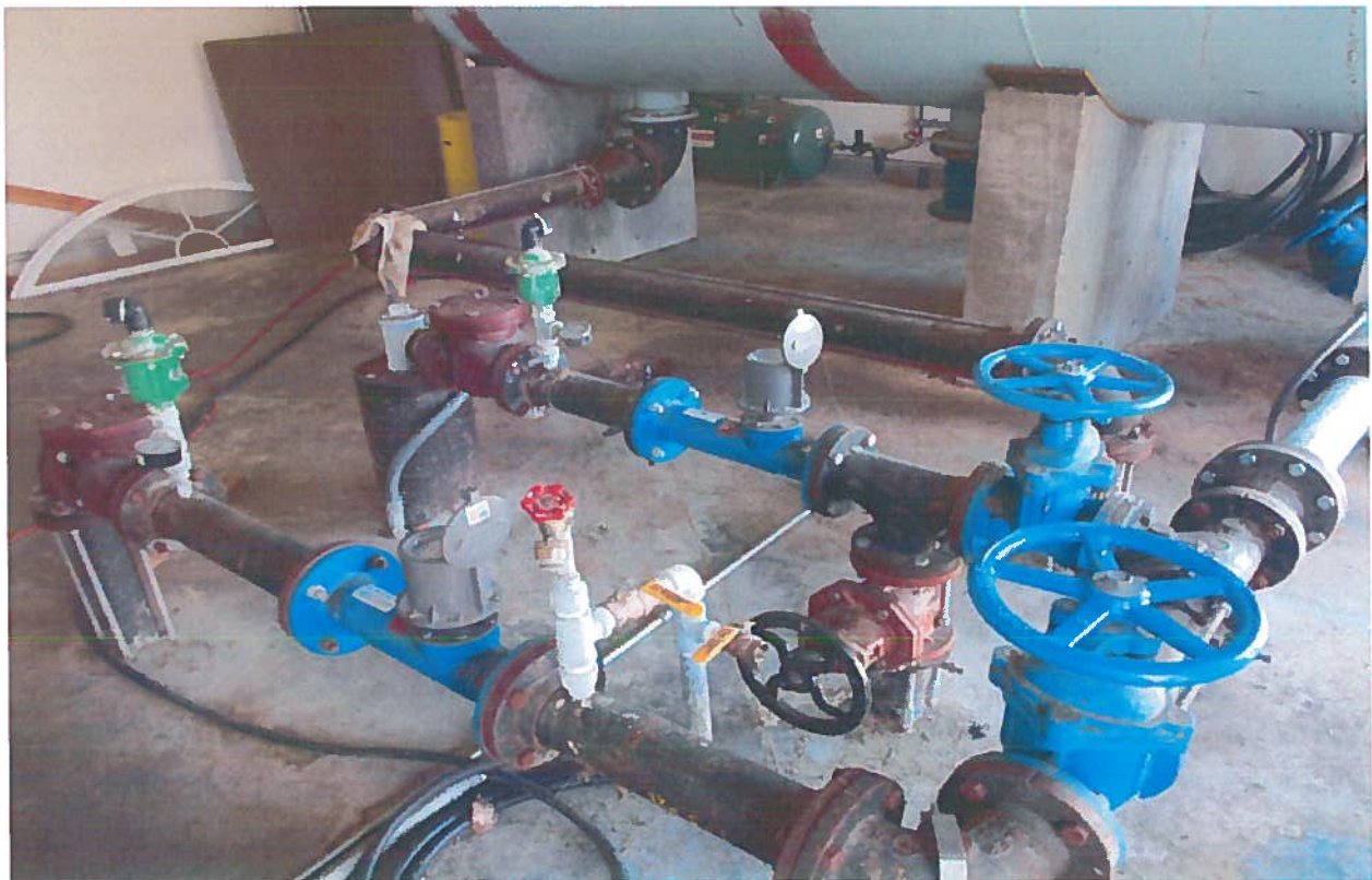
Plumbing inside wellhouse
