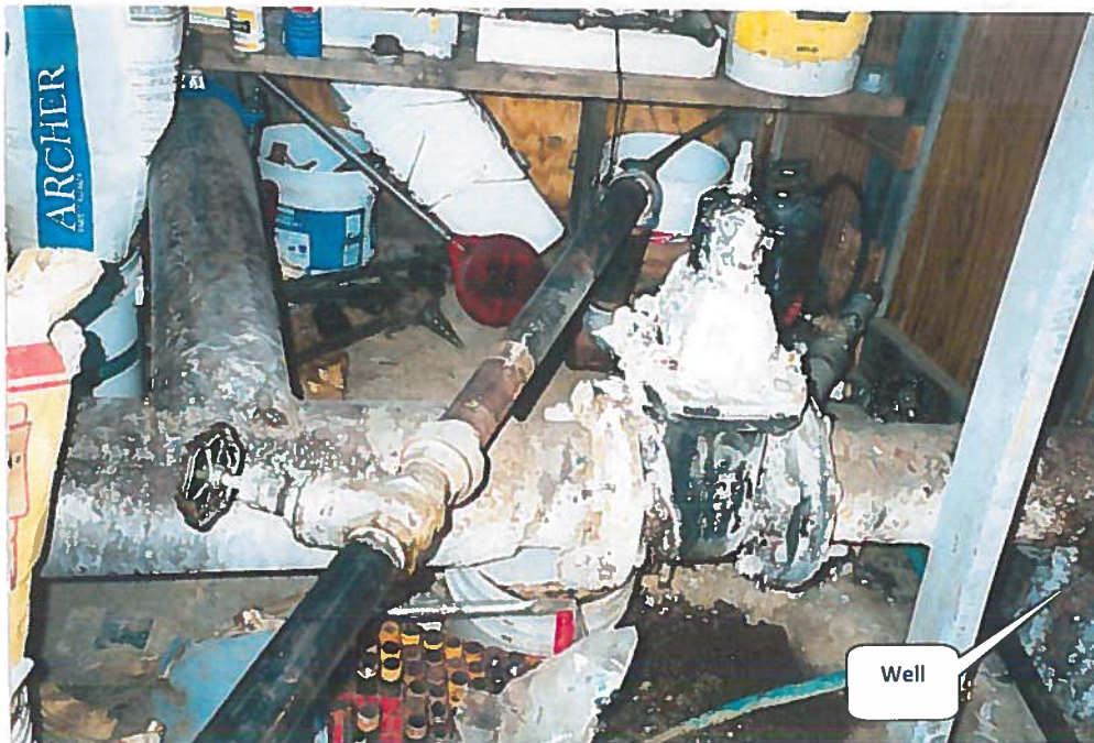
LEFT: View on January 8, 1999 of the 47-7520 well (right edge of photo) and plumbing system. Note that the plumbing system had been modified when this picture was taken. Also note that the well is now located inside a small building (compared to 1992 photo above)
