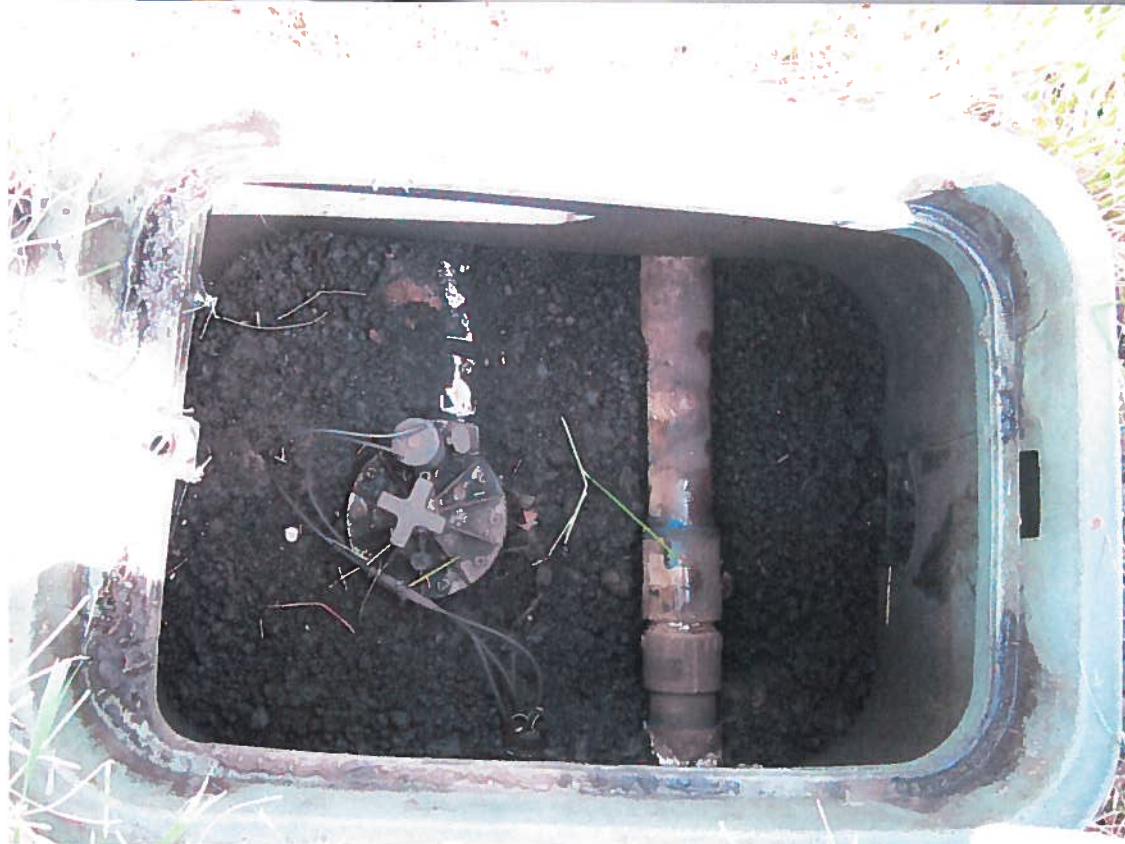
Sprinkler box within POV
