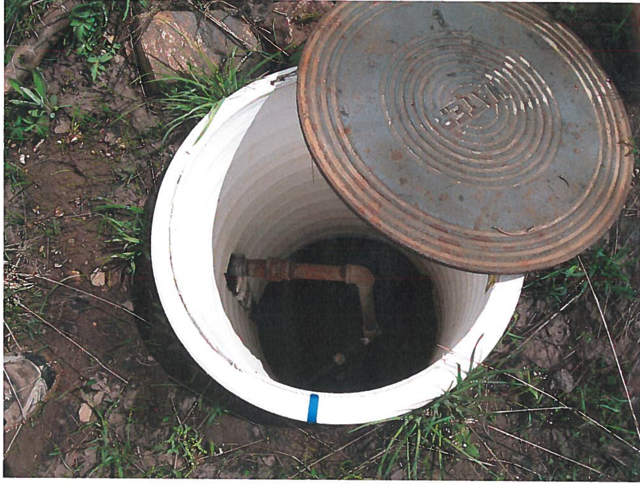
Valve at group site for stock trough line
