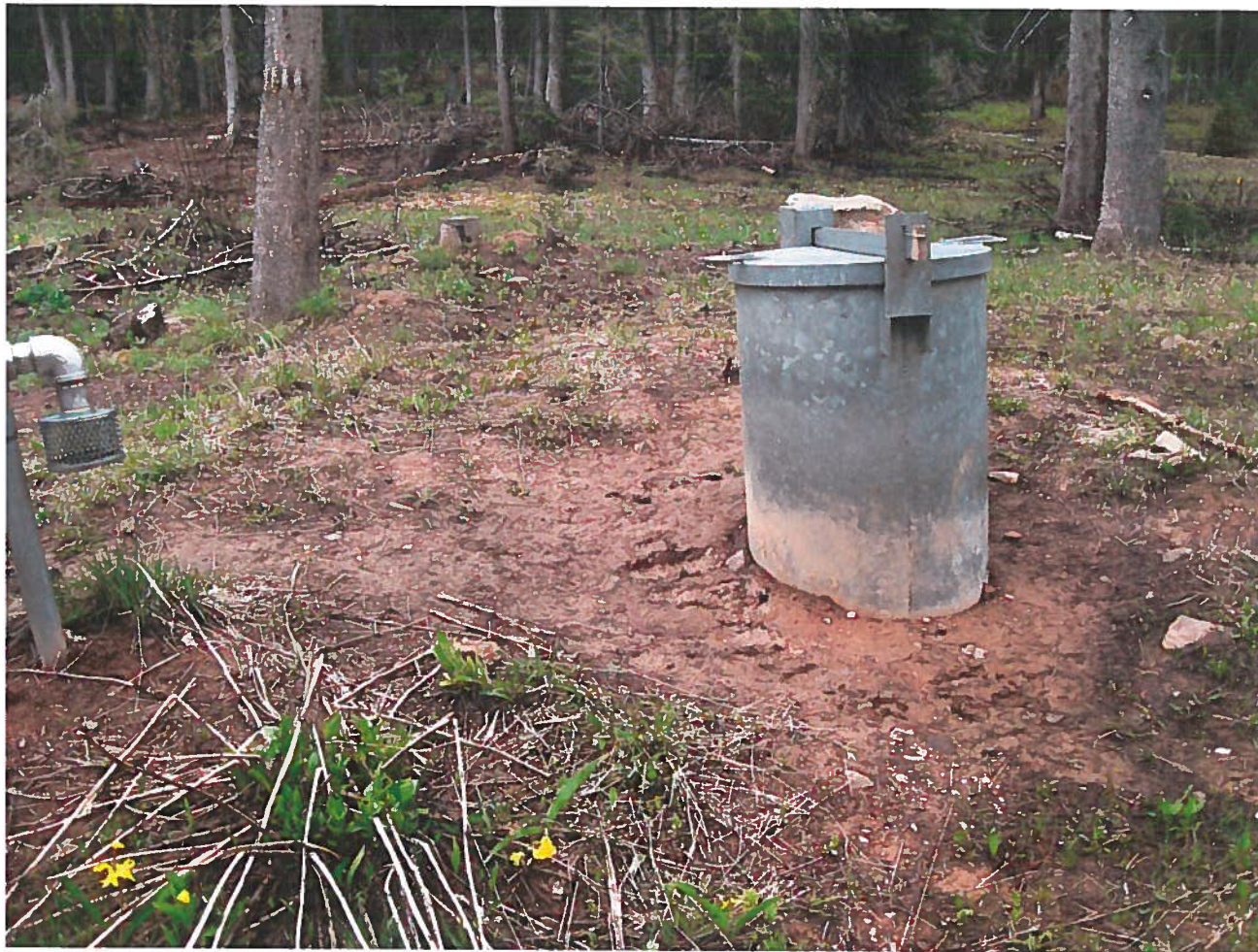
top of 10,000 gal tank
