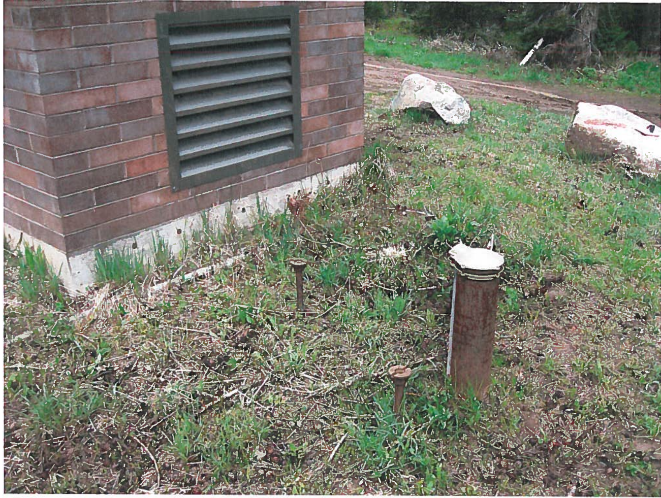
Well head near pump house
