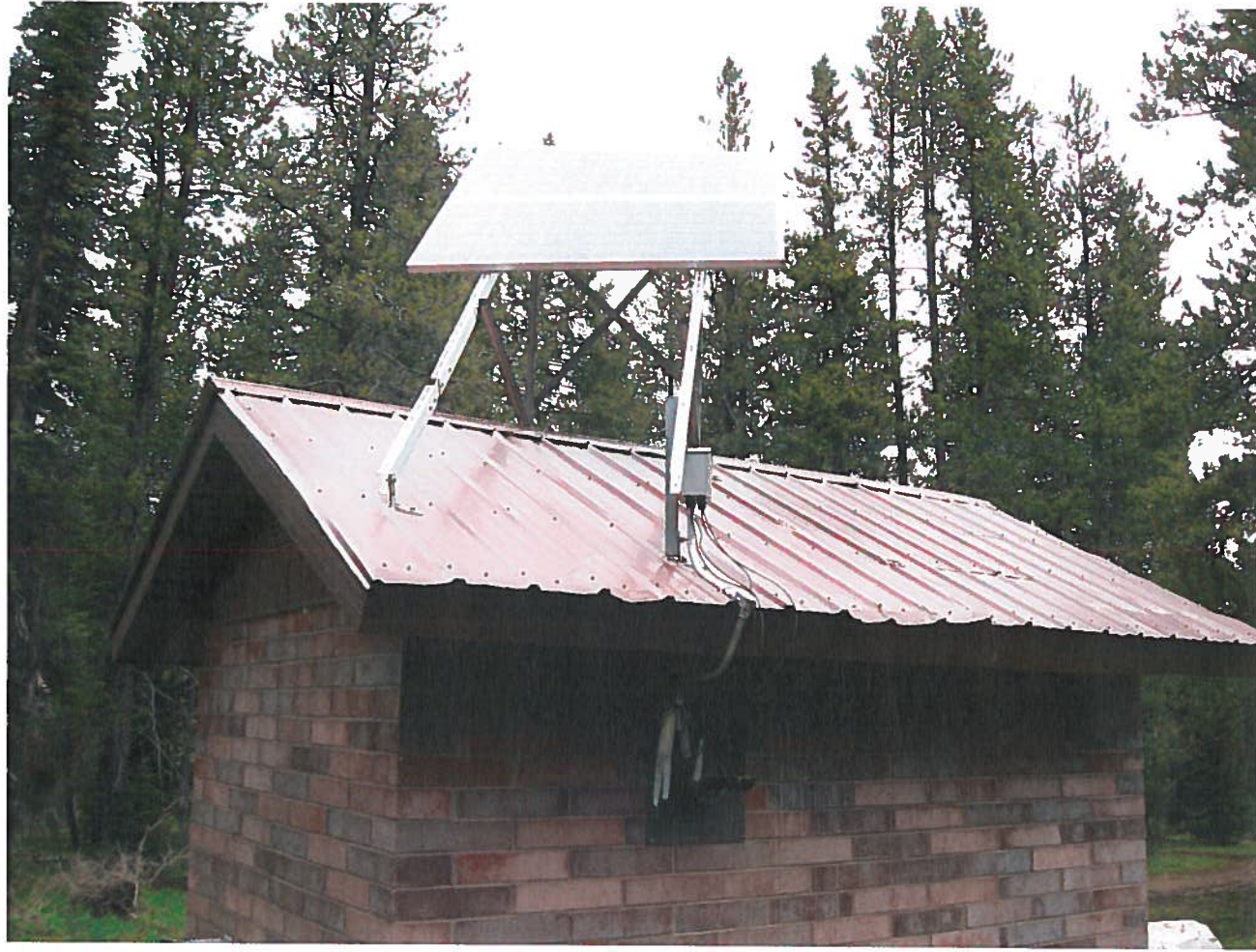
Solar panels on pump house
