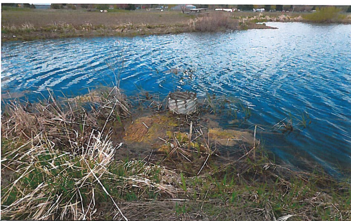
Place of Use: View westerly of the screened 18" CMP overflow stand pipe. The 18" CMP overflow stand pipe is not active during normal filling of the recreation storage pond. It is only used during emergency situations.
