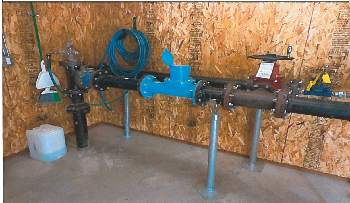
View inside of pump house/mechanical building of the 4" steel supply line from the well and the 4" steel discharge main line providing water to the 45 lot North Ridge at Terrace Lakes development. The 4" discharge line expands to 6" approximately 50 feet from the pump house/mechanical building.
