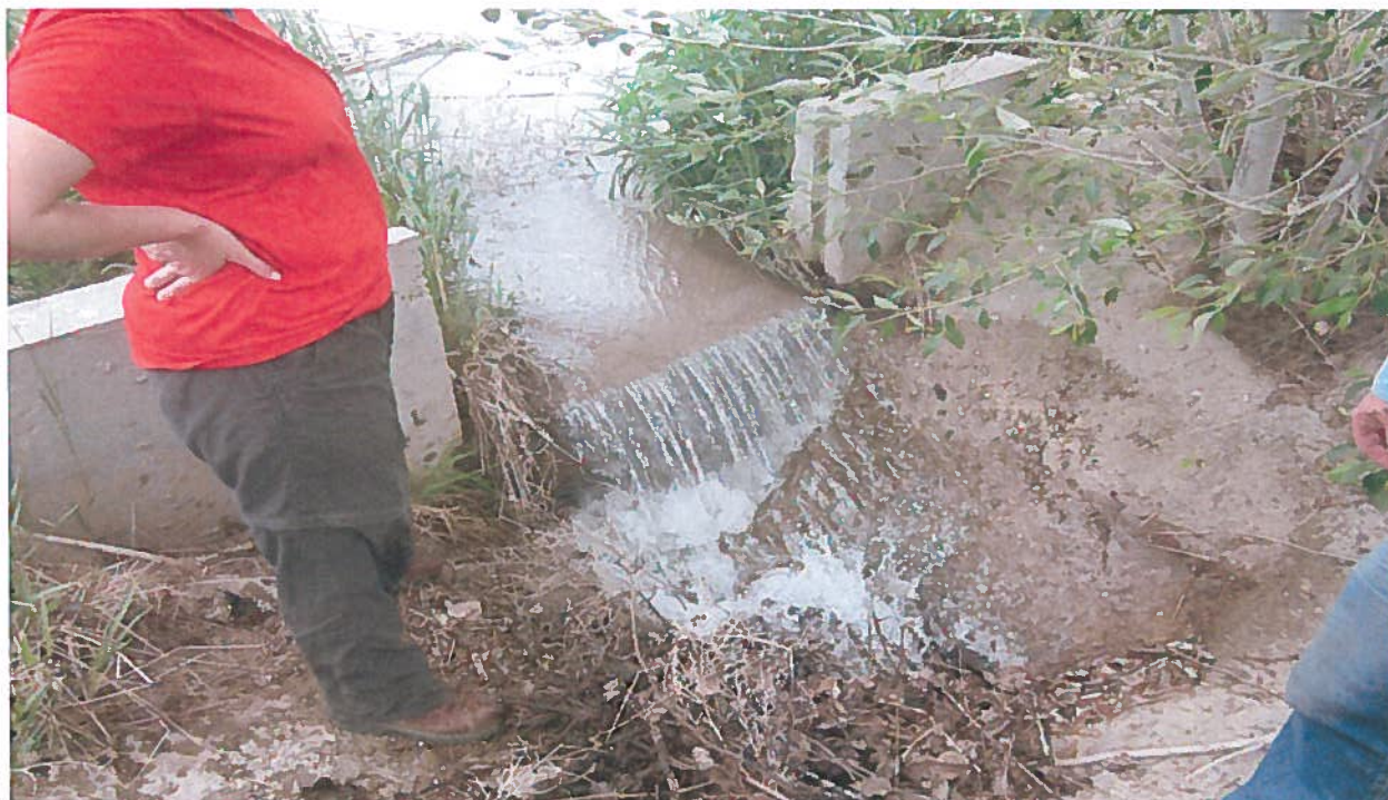
A weir at the pond overflow, in the southwest corner of the pond. The overflow water discharges through a drain into the creek that was tiled many years ago.
