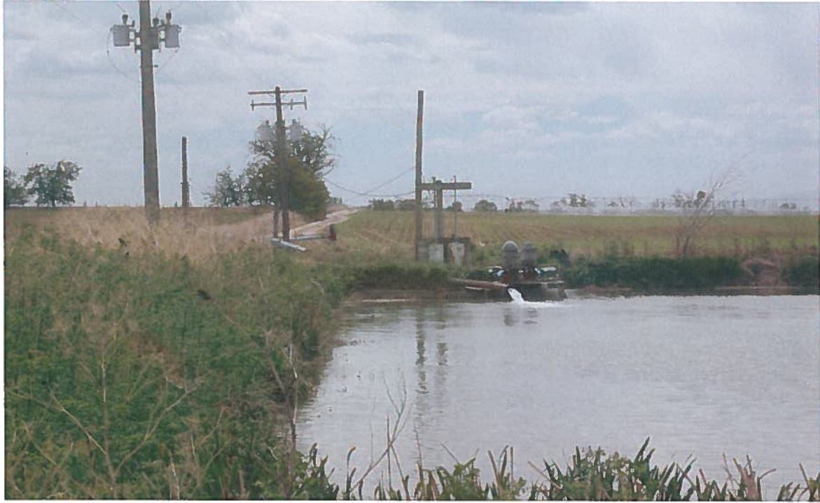
The pump station seen, with the 50 hp and the 75 hp turbines.
