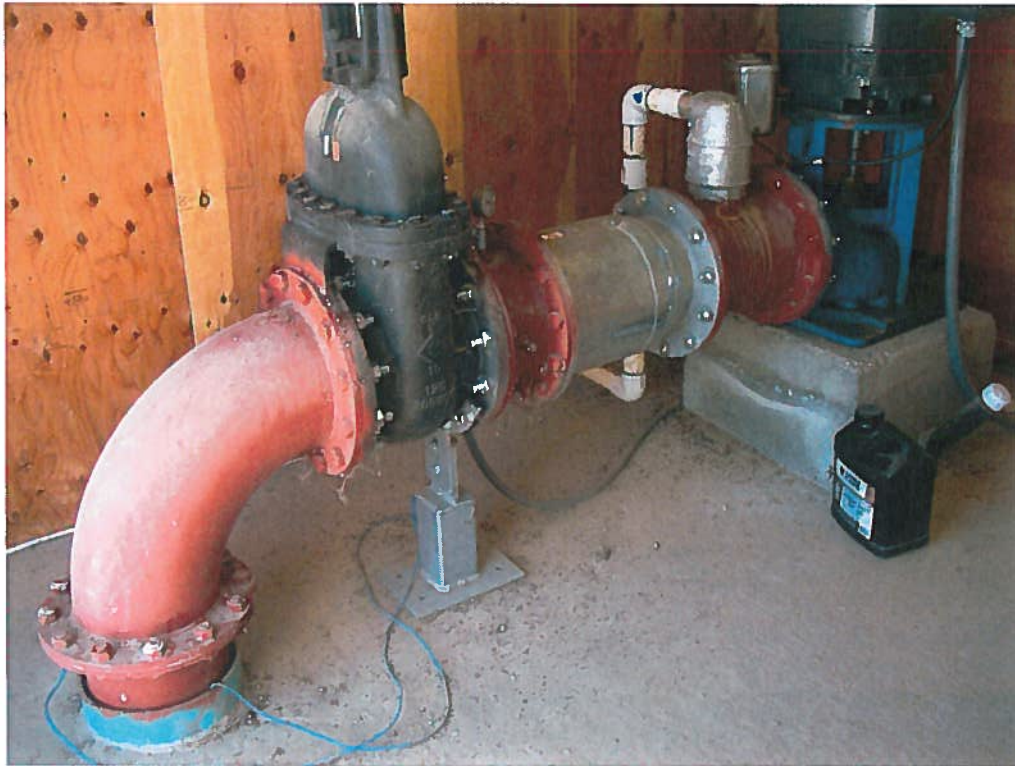
63-31995 Exam 8/24/2012: POD well and motor with 10 inch discharge inside pump house.
