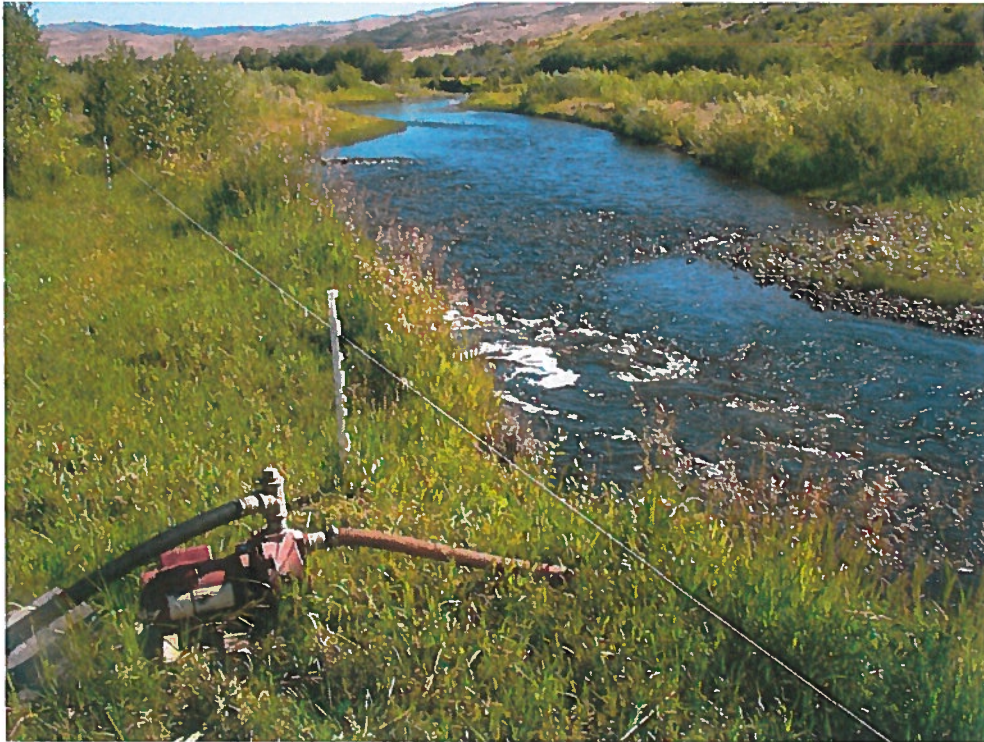
65-13968 Site Visit/Exam 6/28/2013: POD pump with 2 inch diameter discharge facing north.
