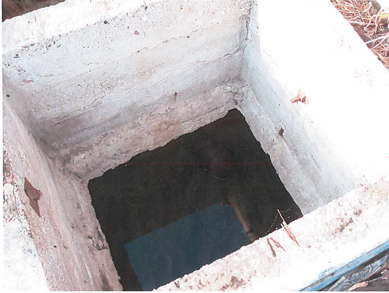
Spring box, full of water, overflow pipe visible
