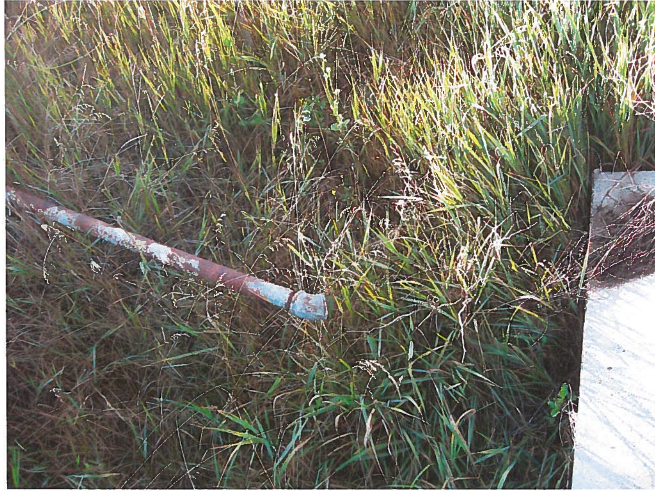
metal pipe running to house - cut at spring box
