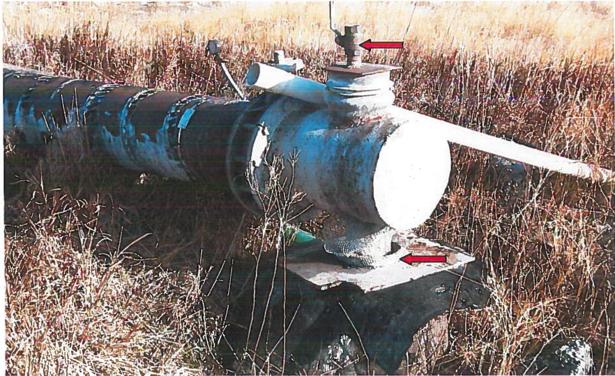
Injection Wellhead – Air is drawn into well at points shown by arrows
