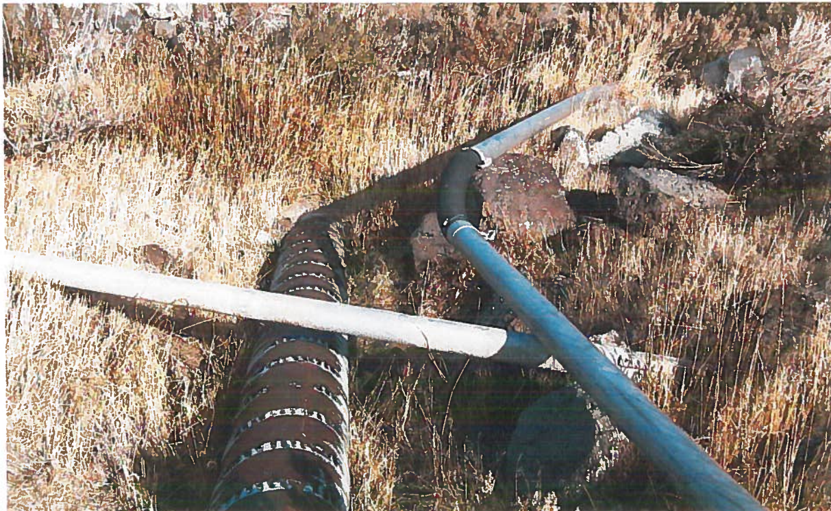
Incoming waterline(left) and outgoing compressed air pipeline(right)
