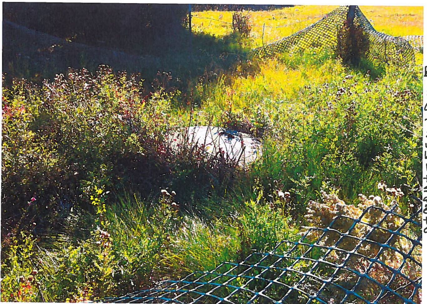
Domestic spring collection tanks 2' x 6' with buried 1/4" PVC that splits 1 goes to each of the 2 cabins
