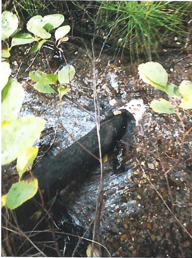
Pipeline that conveys water to the pump house
