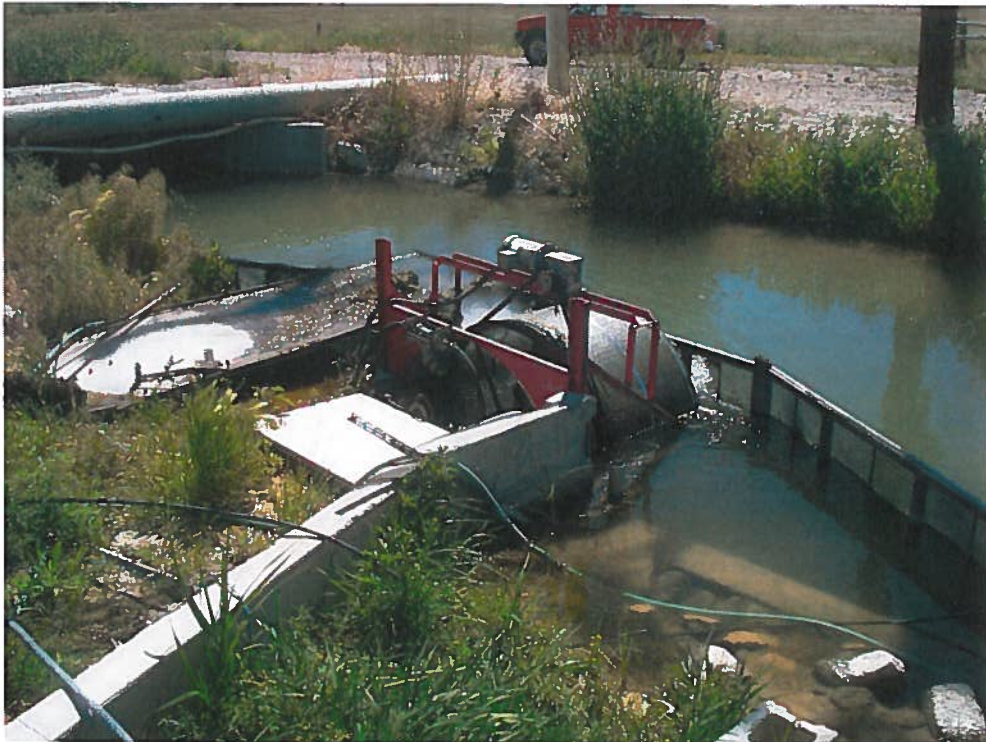
2-7431 Exam 6/4/2013: Water wheel/screen inside ditch at Wastewater POD. Water through screen goes into vault from which three motors/pumps pull water. Downstream weir in photo background. Upstream weir outside of photo.
