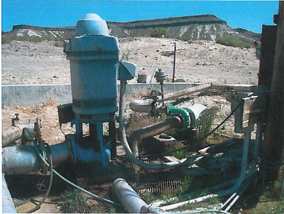
2-7431 Exam 6/4/2013: Wastewater POD 100 hp turbine motor/pump and 30 hp motor/pump. 20 hp motor/pump just outside of photo view in foreground. 4 inch line in photo background diverts water to reservoir.
