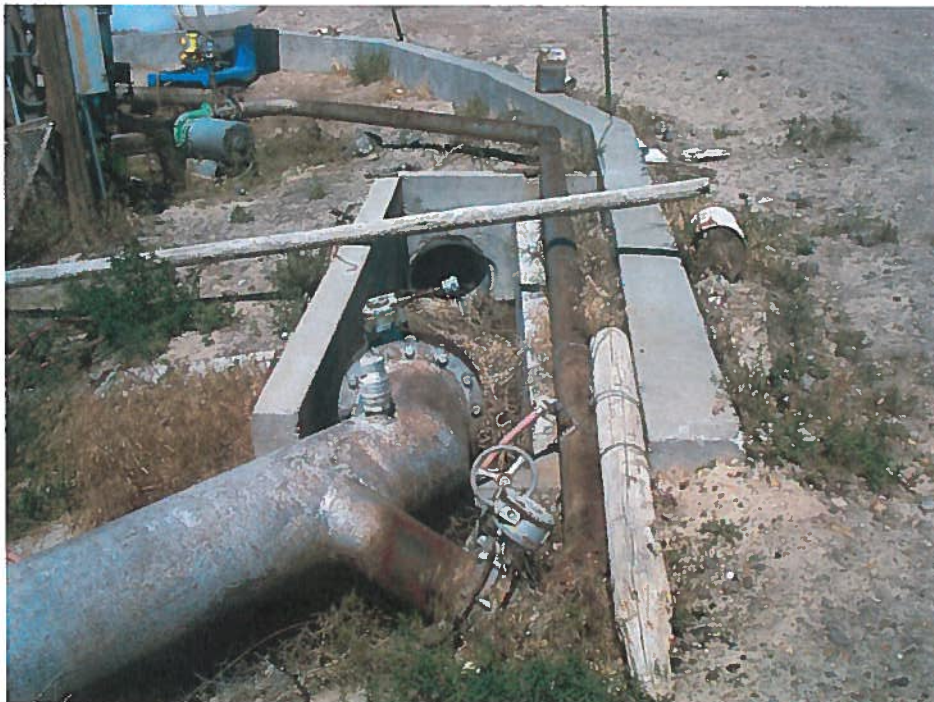
2-7431 Exam 6/4/2013: Location where 14 inch line from Snake River POD intersects 4 inch line from Wastewater POD connects to 4 inch line diverts water to reservoir.
