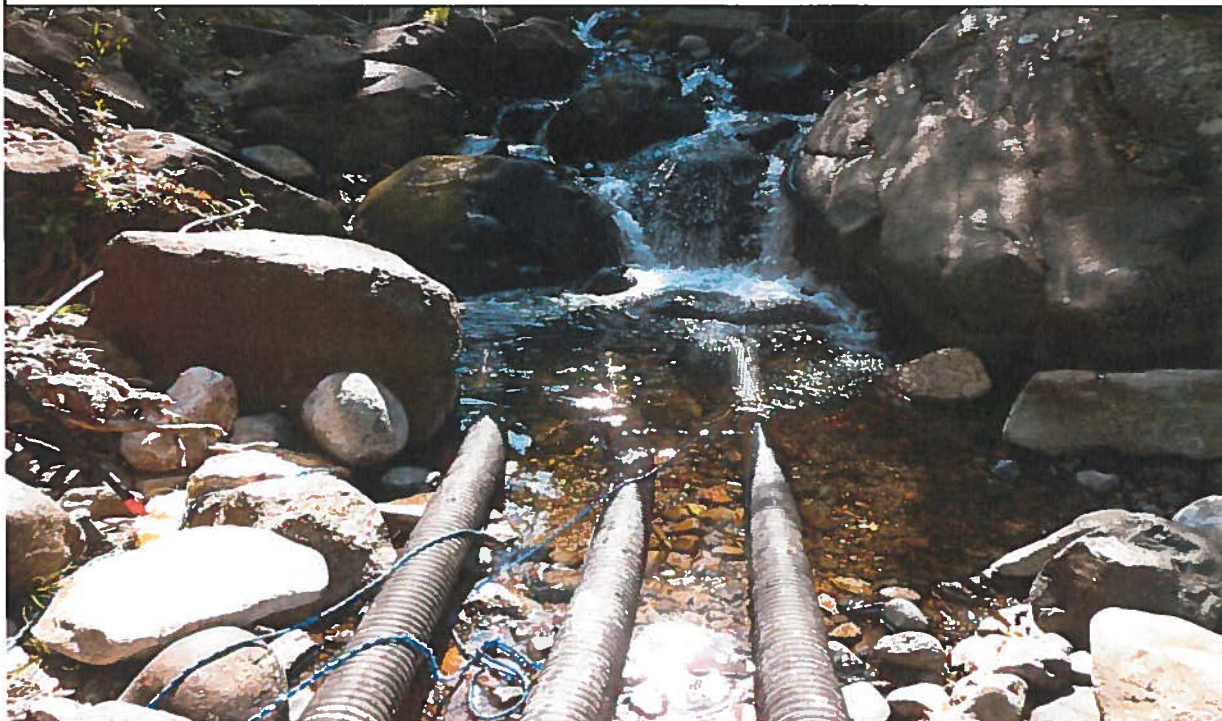
Point of Diversion: View southeasterly of three (3) 5" diameter flexible suction pipe in Hat Creek. A metal intake screen is attached to the end of each 5" diameter flexible pipe.
