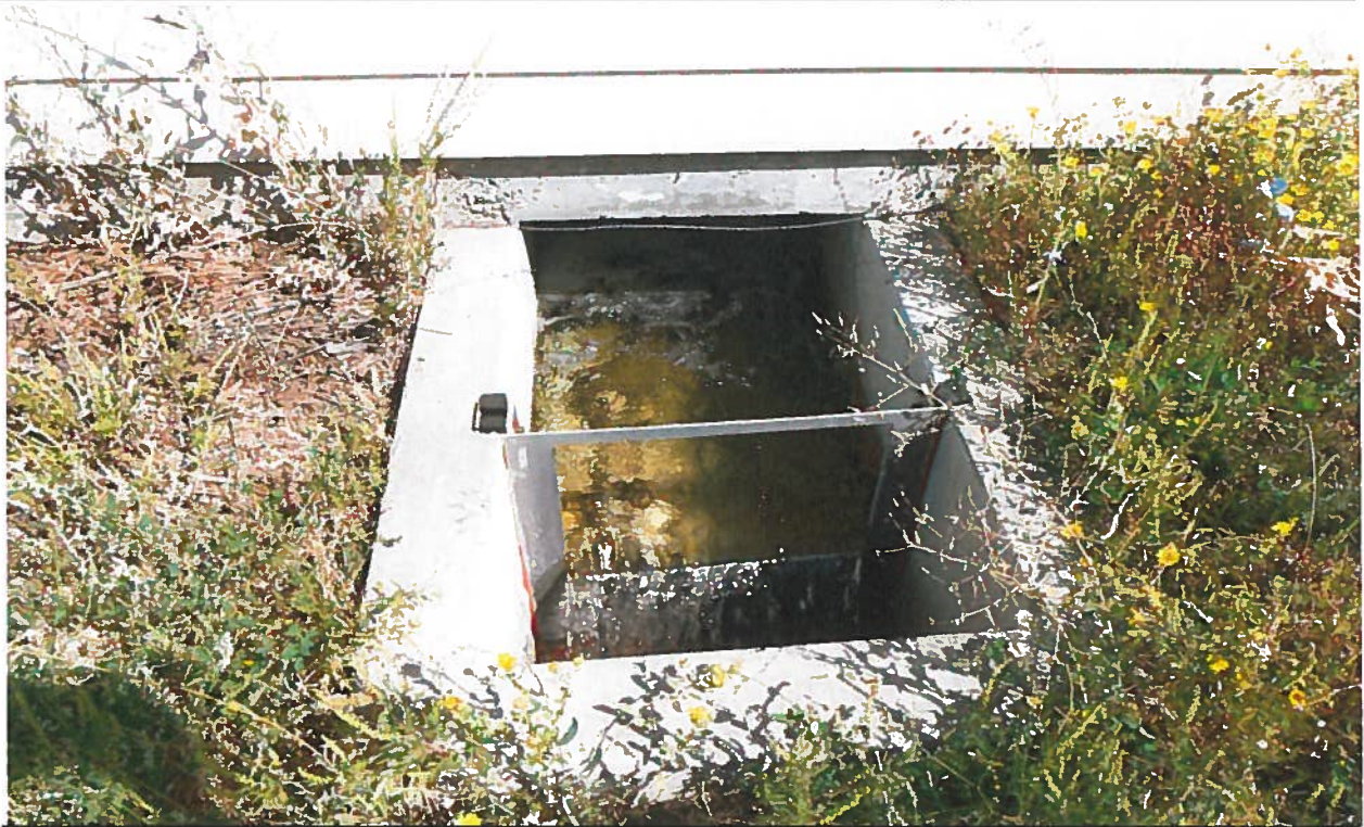
View northerly of tail race located on the south side of the power station. The tail race diverts water to a 12" PVC pipe for discharge back to Hat Creek. An 18" wide by 15" high rectangular weir has been installed in the tail race for measurement of the discharge back to Hat Creek.
