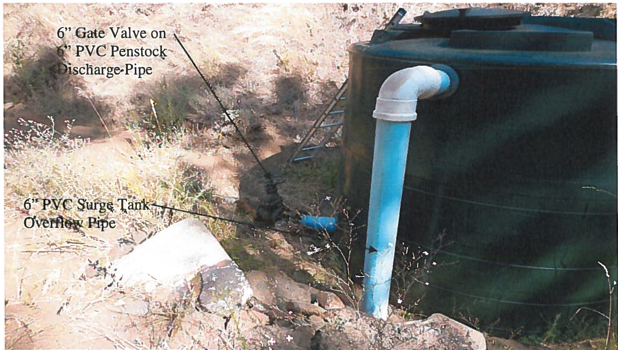
View northwesterly of 3000 gallon surge tank, 6" PVC overflow, and 6" gate valve on 6" PVC penstock discharge pipe.
