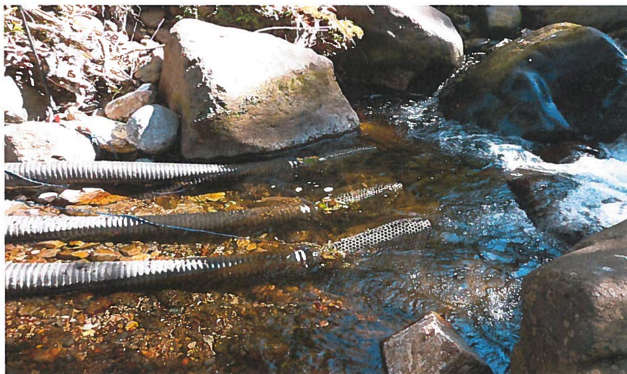
Point of Diversion: View northeasterly of the intake screens attached to the three (3) 5" diameter flexible suction pipes in Hat Creek.
