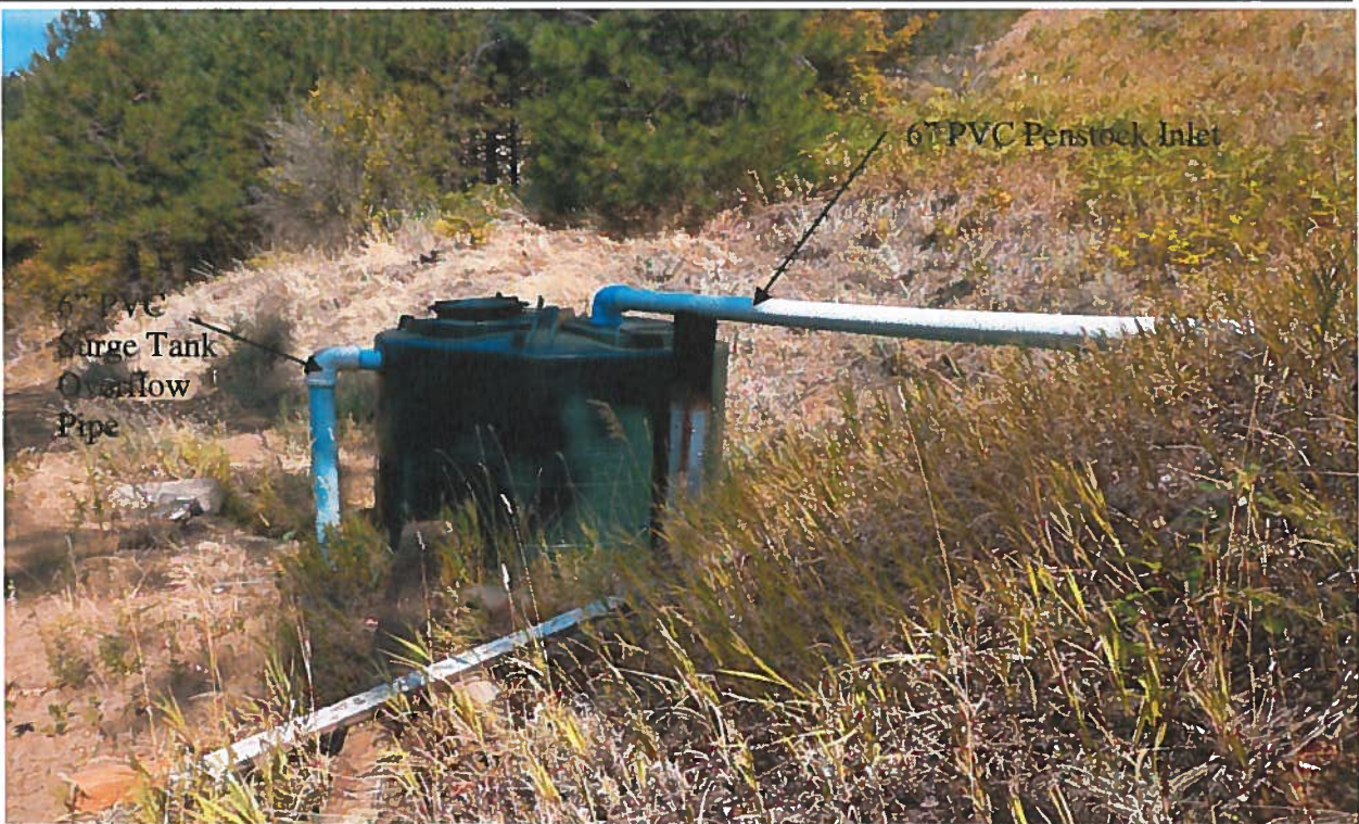
View northwesterly of the 3000 gallon surge tank located approximately 350 feet northwest of the point of diversion. The 6" PVC penstock inlet pipe discharges into the top of the surge tank. The 6" PVC overflow pipe discharges near the top of the surge tank discharges back to Hat Creek.
