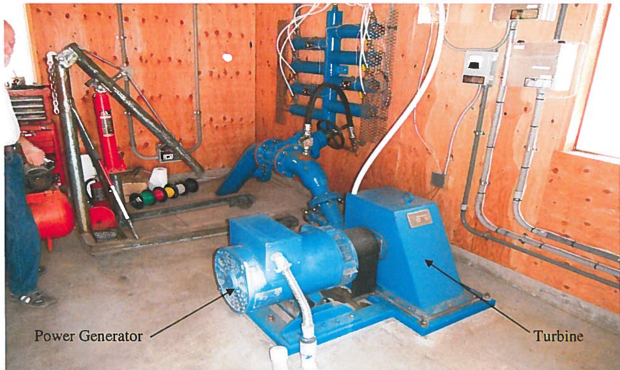
View inside of power plant of 6" steel penstock discharging to turbine. A concrete tail race is located below the turbine for discharge to 12" PVC for discharge back to Hat Creek.
