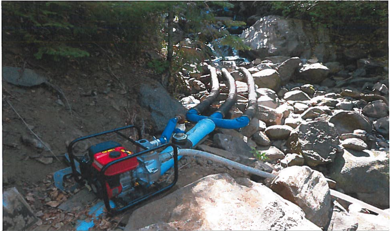
Point of Diversion: View southeasterly of a 5" steel manifold discharging to the 6" PVC penstock. A portable pump and generator with a 2" flexible suction and discharge pipe in foreground is used for charging the three (3) 5" diameter flexible pipes.
