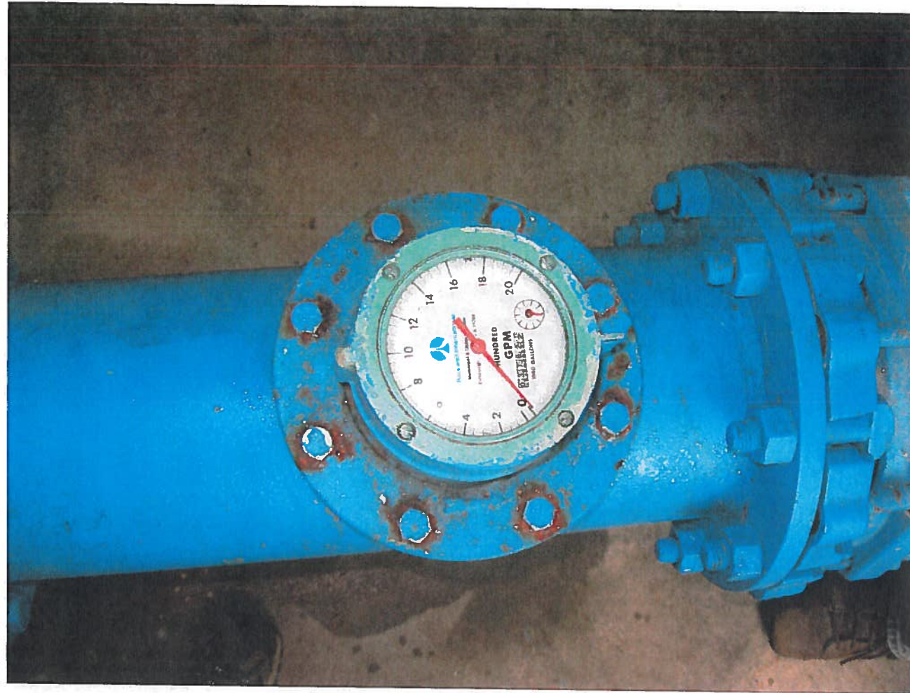
Flow meter on Well #2
