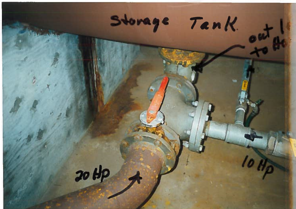
Showing inlet from from 20 Hp pump and 10 Hp pump, storage tank and outlet to System.
