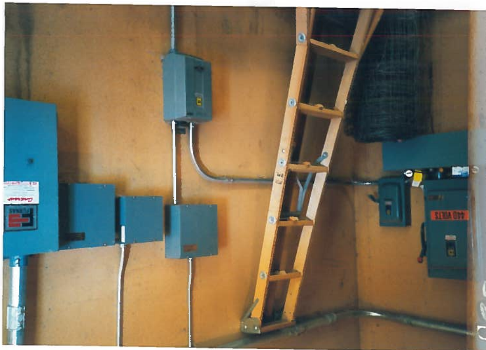
Pump Control Boxes on East and South walls Permit # 27-7581
