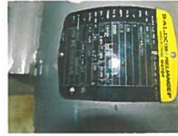
WELL PUMP .JPG
