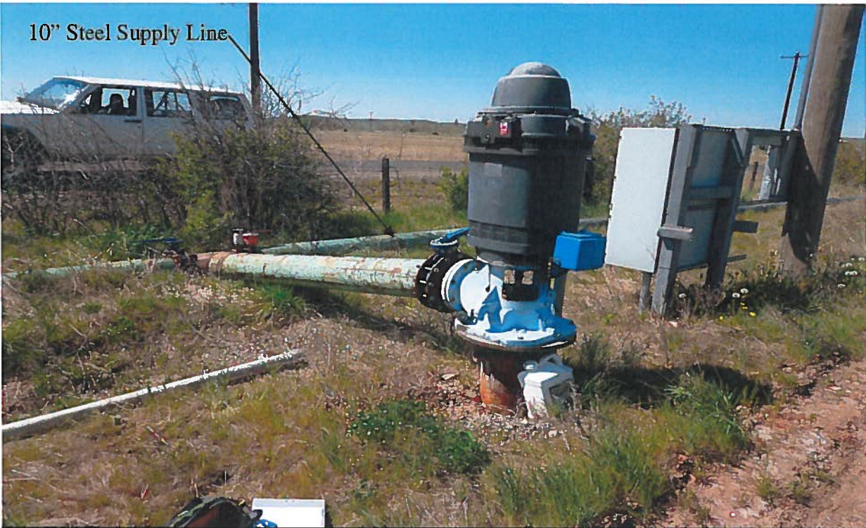
Point of Diversion: View southwesterly of the well and vertical turbine pump located near Grays Creek Road. The well discharges ground water to the 10" steel supply line which parallels Grays Creek Road. Water is diverted to a collection and pumping basin for discharging to the place of use to operate the 'Blue' and 'Yellow' pivot irrigation systems.
