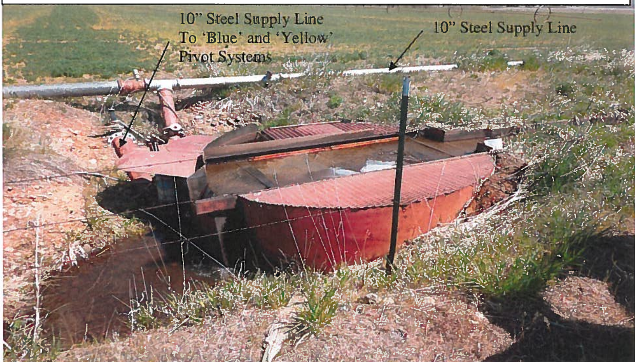
View northerly of a collection and pumping basin for surface water from the Little Weiser Irrigation District. Water is pumped through a 10" steel supply line to the north to operate the 'Blue' and 'Yellow' pivot systems. Well water is discharged to the collection and pumping basin when surface water is not available.
