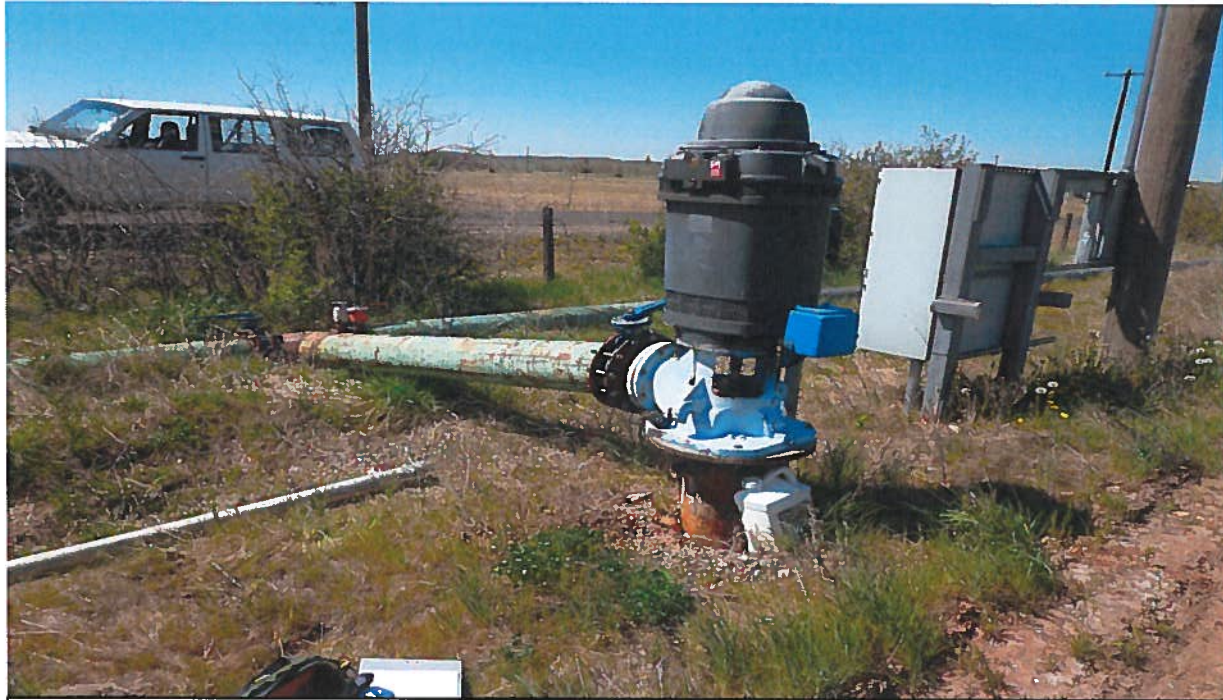
Point of Diversion: View southwesterly of a well and vertical turbine pump located near Grays Creek Road. The well discharges ground water to the 10" steel supply line which parallels Grays Creek Road. Water is diverted to a collection and pumping basin for discharging to the place of use to operate the 'Blue' and 'Yellow' pivot irrigation systems.
