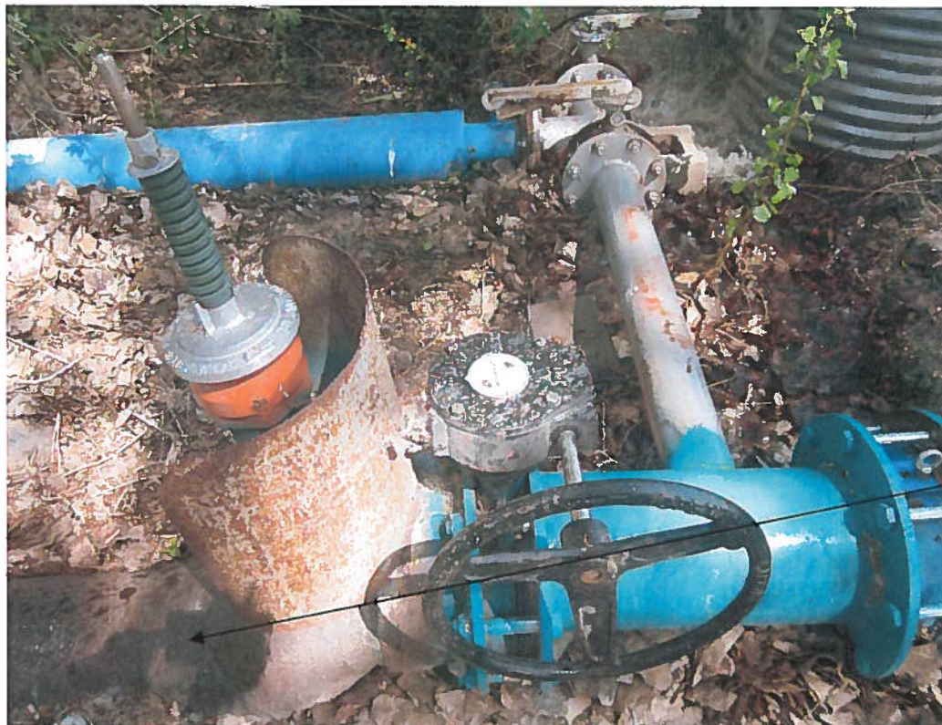
8" buried pipe to distribution system
