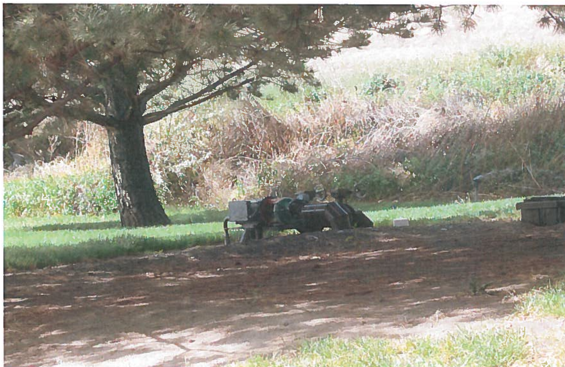
Booster pump located in the irrigated common area
