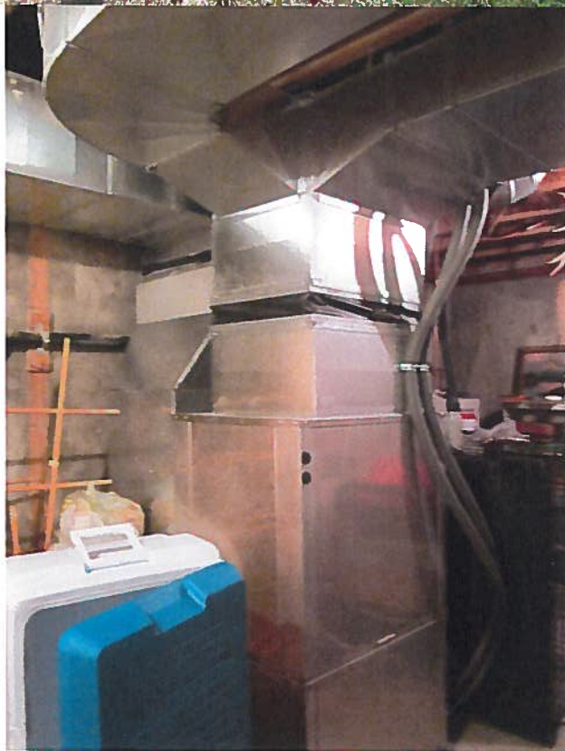
Heating/cooling system in the home's basement
