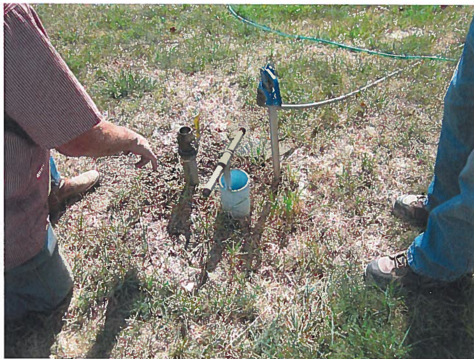
Hydrant and irrigation hydrant
