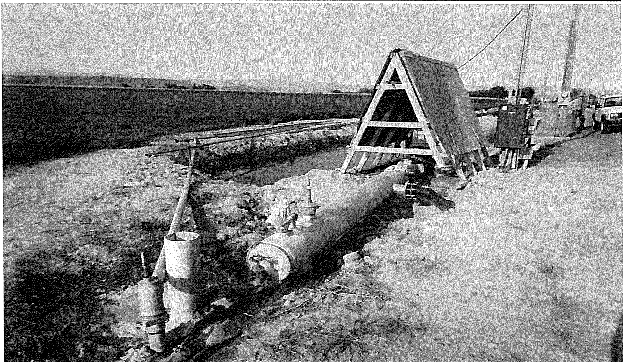
Irrigation Pond Pump Station: View westerly of the irrigation pump station for the long narrow irrigation pond.
