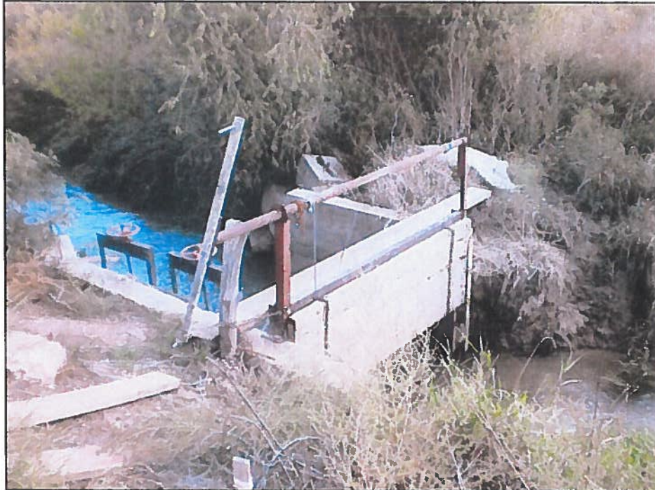
22: Check structure in Baldrige-Meadows Drain. Drain flow is from photo right to left. Headgates supply Lower Haas Ditch.
