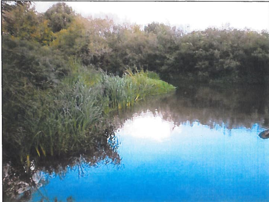
21: Channel below check structure is affected by heavy vegetation growth.
