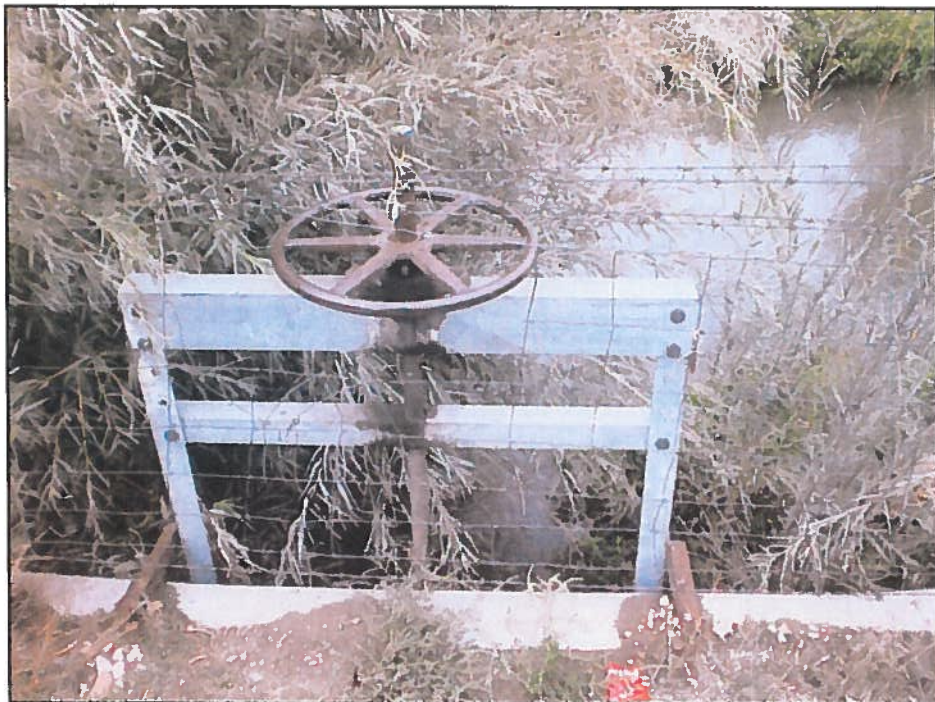
HWY 95: Headgate controlling diversions from Sand Hollow Creek at Highway 95.
