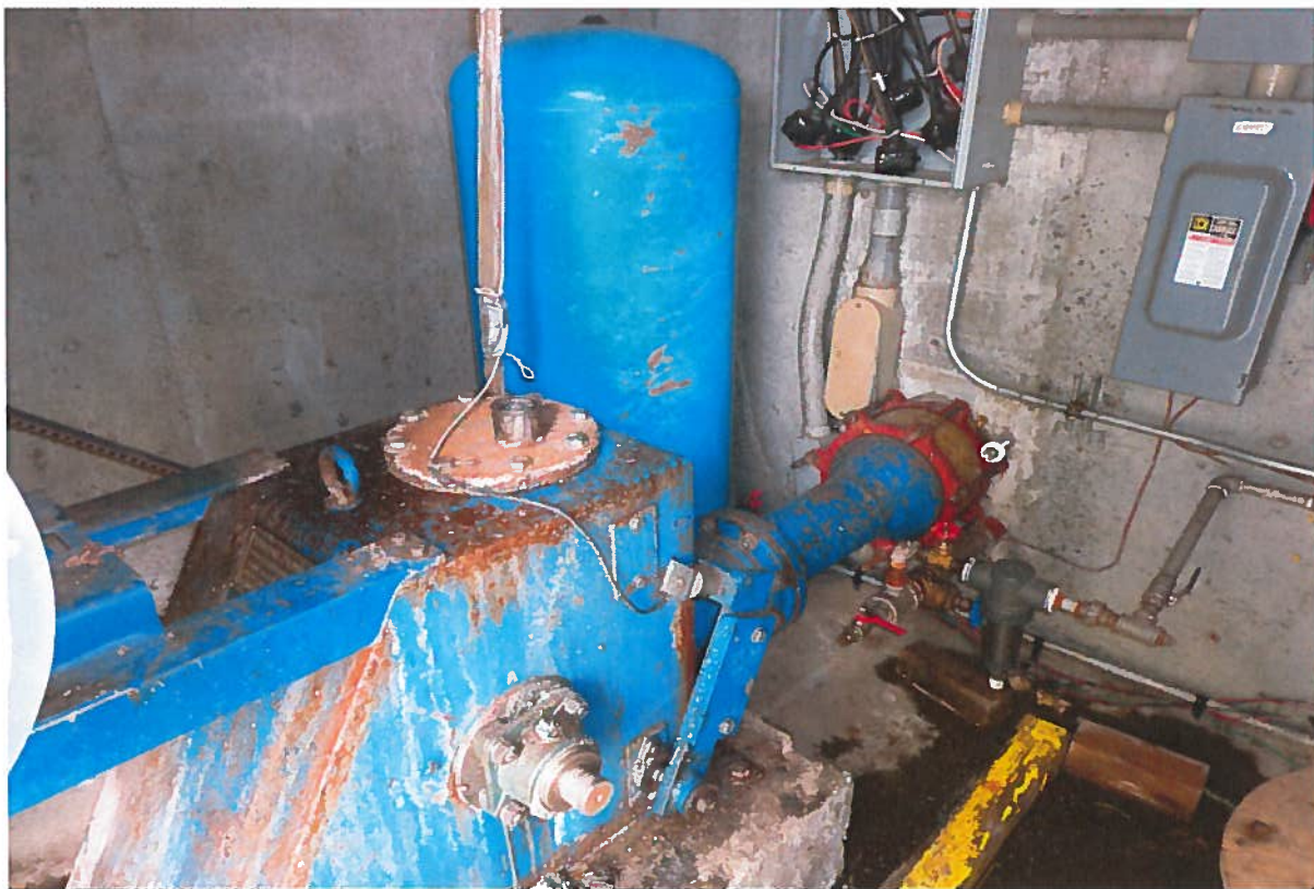
View inside the powerhouse of the 10" penstock reducing to 6" prior to discharging through a 1" diameter orifice to the pelton wheel turbine.
