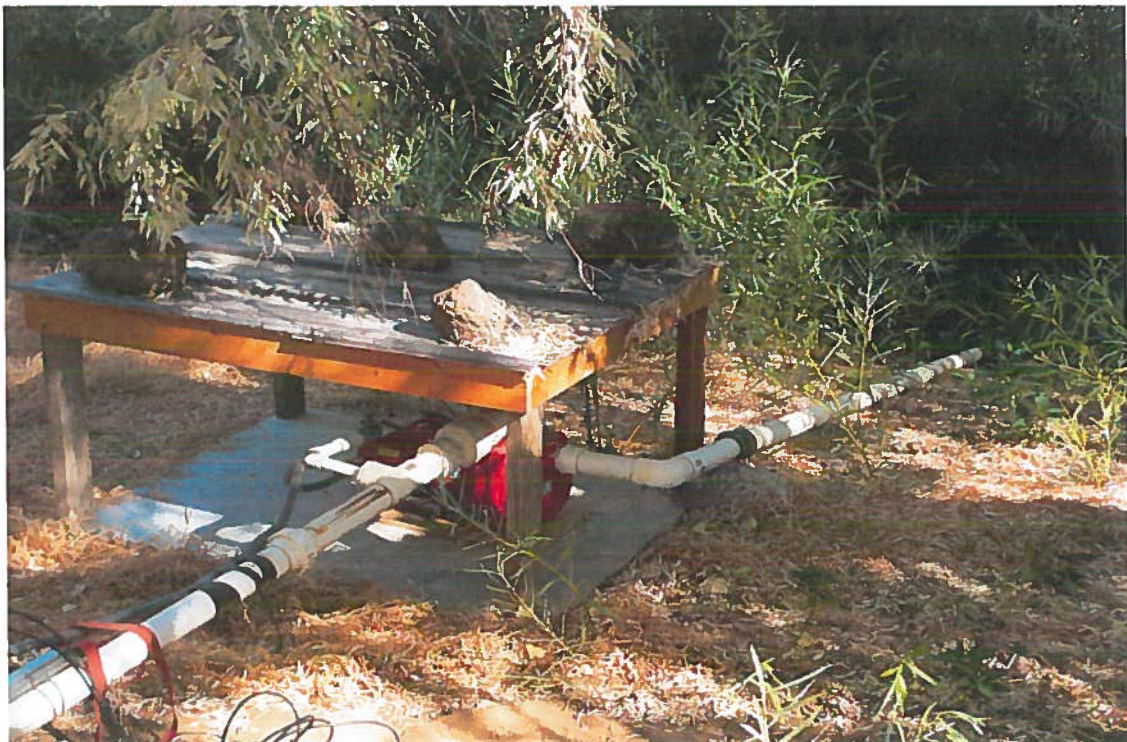
View of Ditch Pump and Pipe Drawing Water from Ditch
