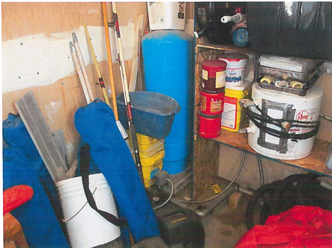
Plumbing Inside Well house
