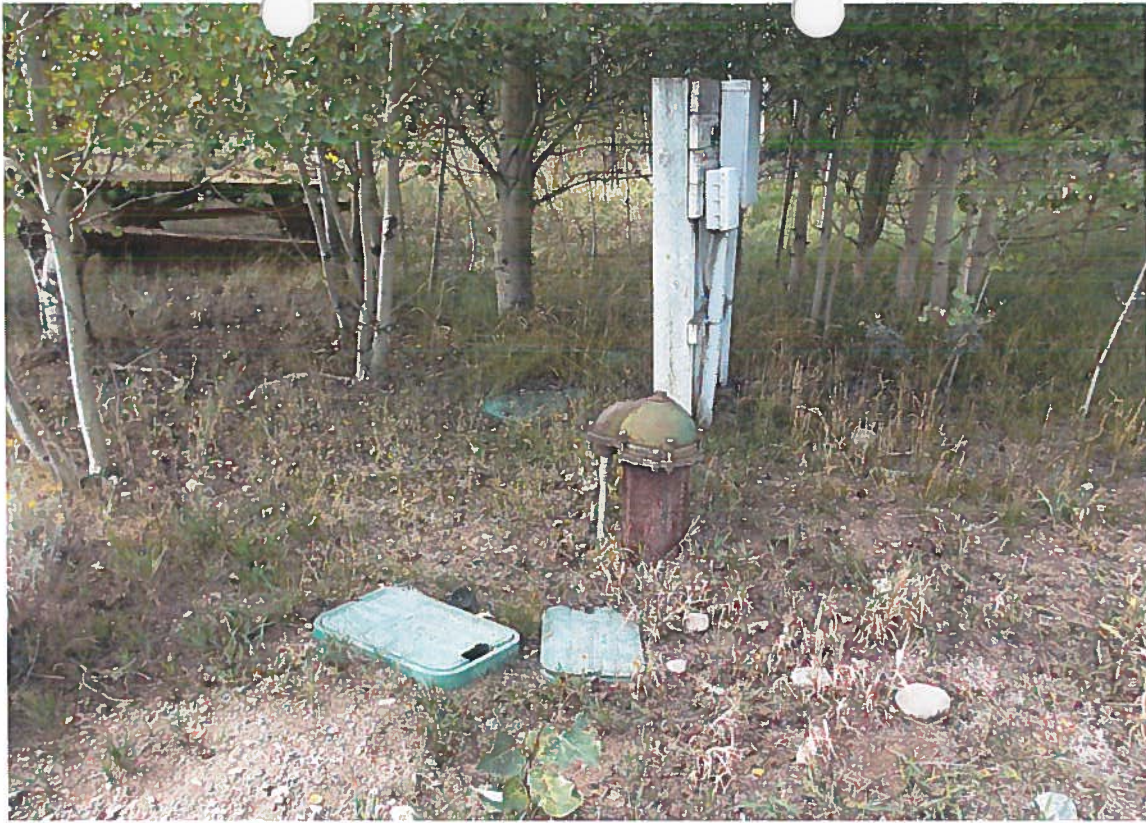
Well and underground control boxes
