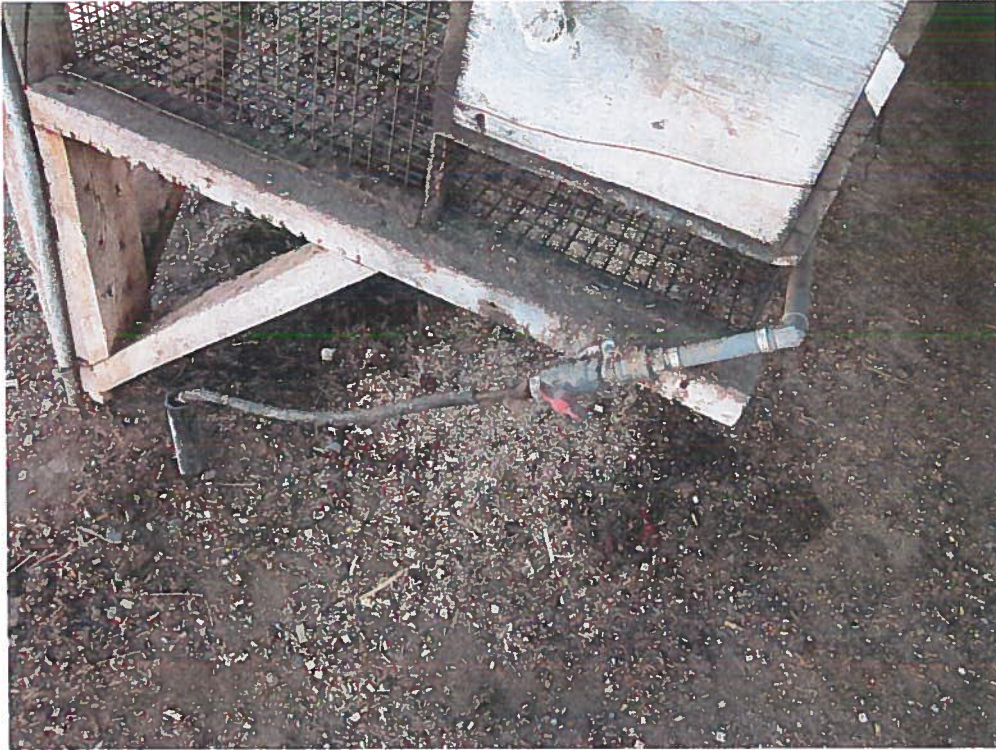
Figure 3: Typical water supply line to trough
