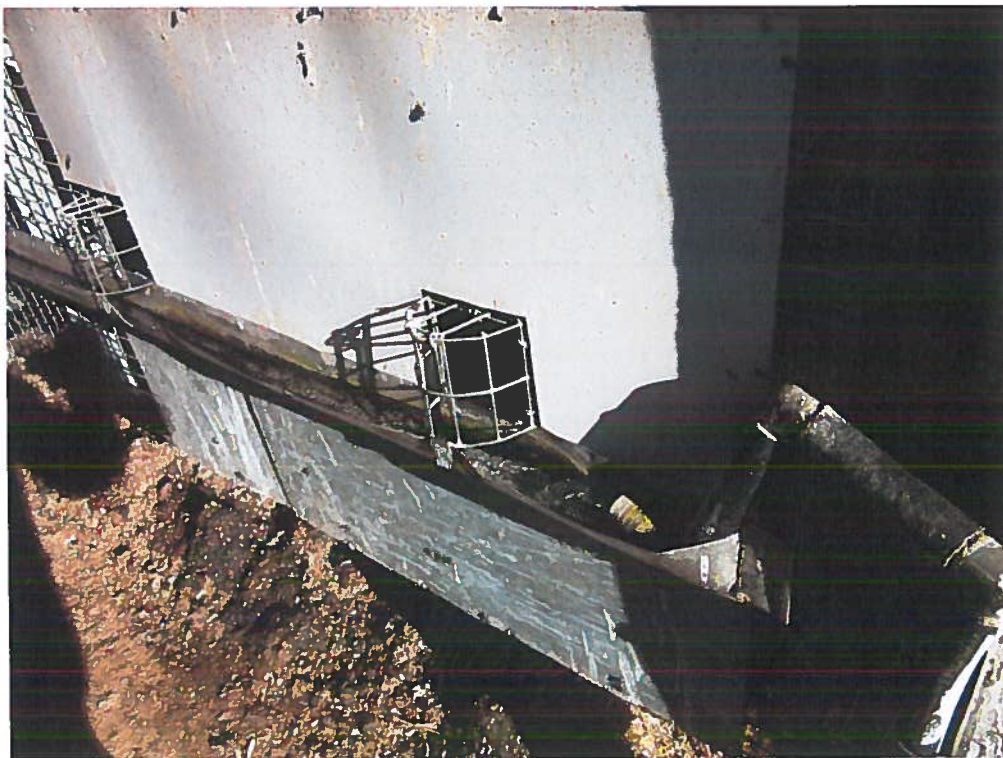
Figure 2: Supply line diverting water into trough
