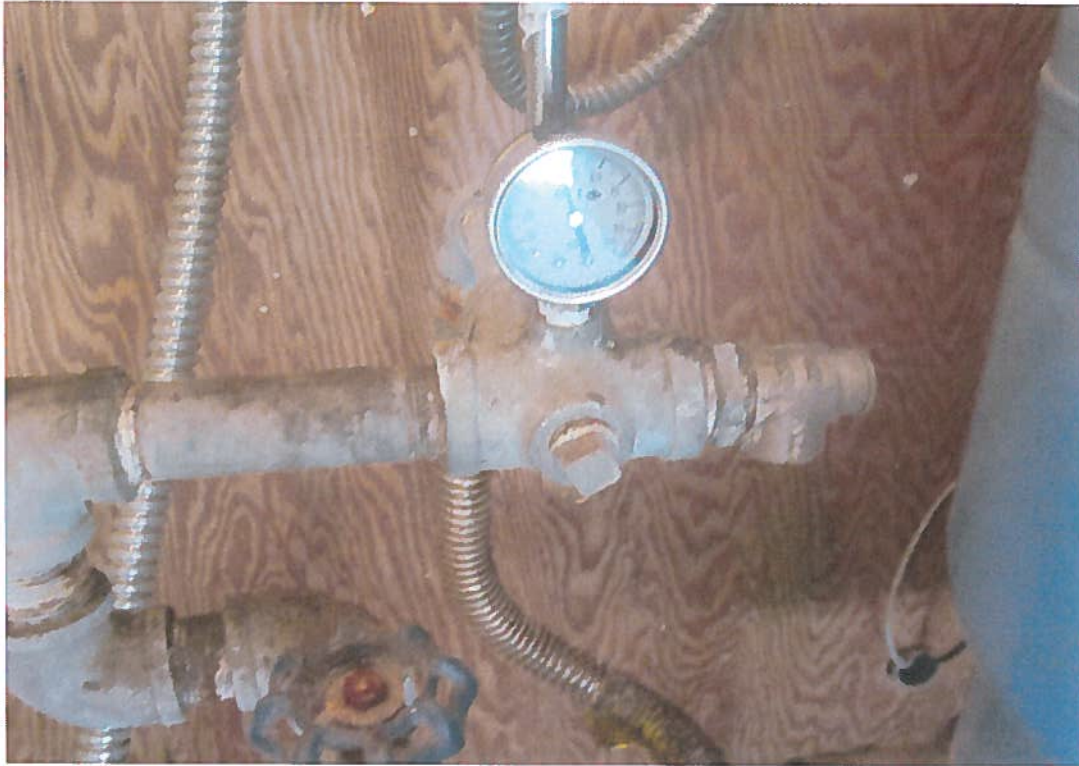
Artesian well is inside the pump house. Pressure gauge on artesian well [point of diversion] piping.
