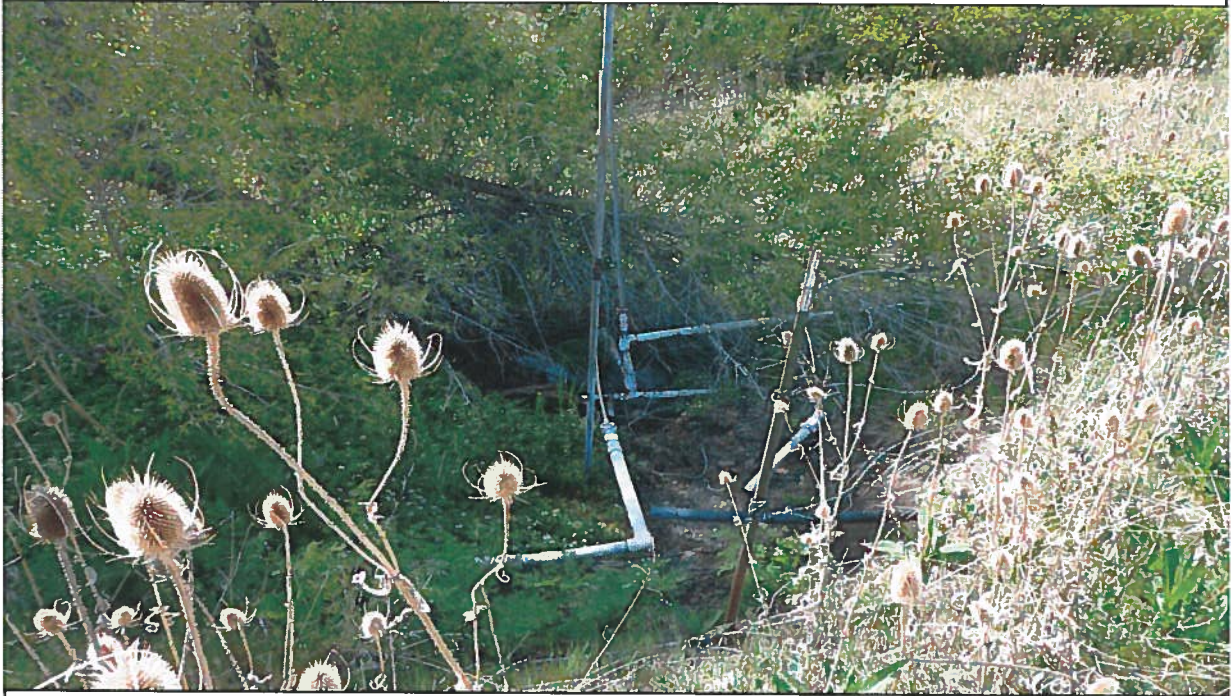
Point of Diversion: View westerly of spring collection and discharge PVC piping located above Storage Pond No.1.
