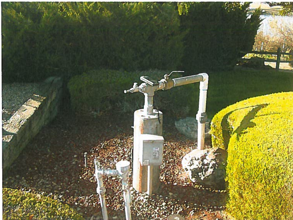
Well with domestic & irrigation pumps
