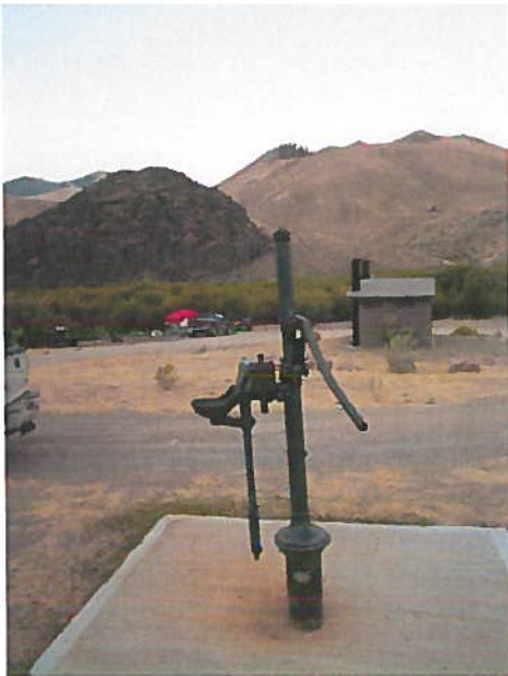
Figure 2. Photograph of POD & POU. Campground is supplied by a single 6" well (D0021741) equipped with a Baker Monitor Handpump.
