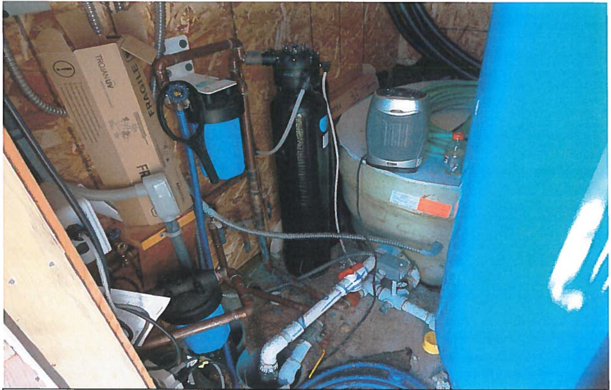
Point of Diversion: View of the 3' diameter plastic pipe spring box and the 1 1/4" PVC discharge piping located in the spring/pump house. The perforated spring box is 12' deep and is encased in drain rock.
