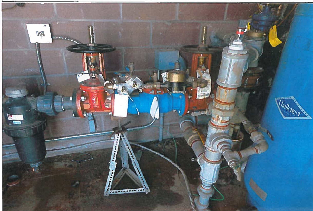
Point of Diversion: View inside of well/pump house of the well, piping, and pressure tank for the school. The piping and appurtenances with the flow meter, gate valve, and filter are associated with the schools pressurized irrigation system.
