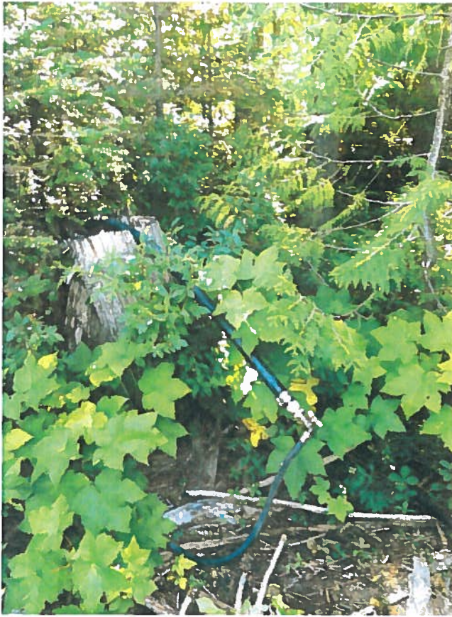
1 1/2 inch poly with hose bib: Test Location at Place of Use
