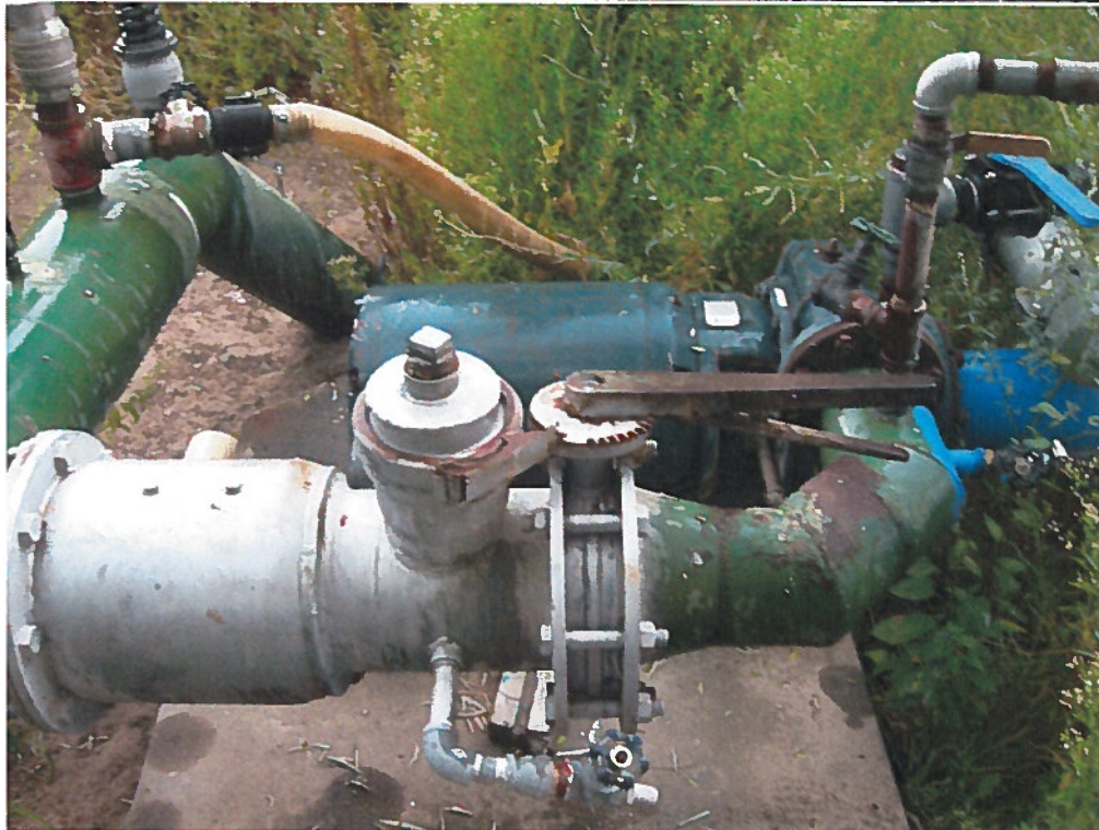
Pump + Motor for PD
