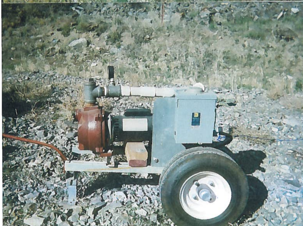
#7C lockable electrical box
