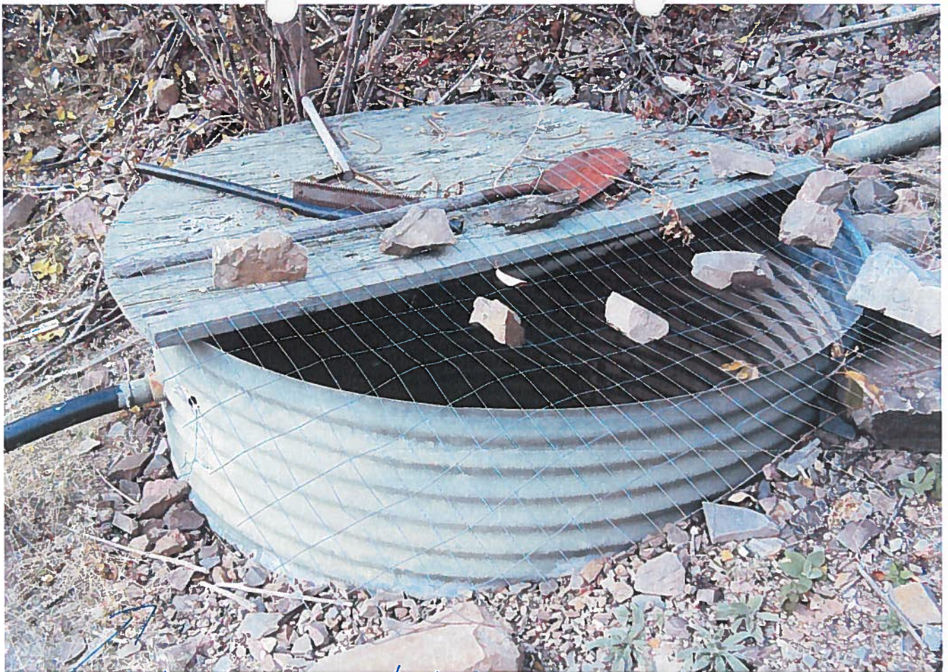
Water collection Tank w/ 2 1/2" line out the top to Gravity feed trees
