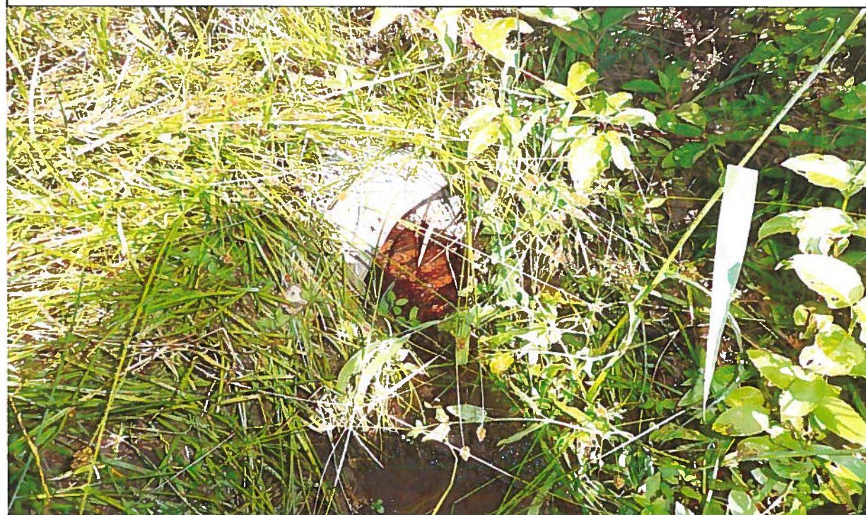
Point of Diversion: View southeasterly of the 10" CMP culvert pipe diverting water from the Unnamed Stream.
