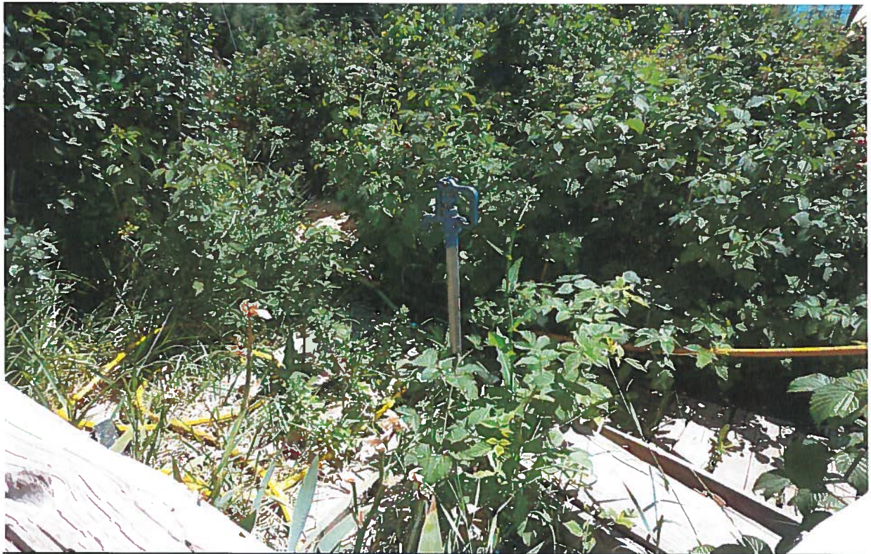
Place of Use: View northeasterly of a frost free hydrant located in the garden area for irrigating the garden and lawn areas.
