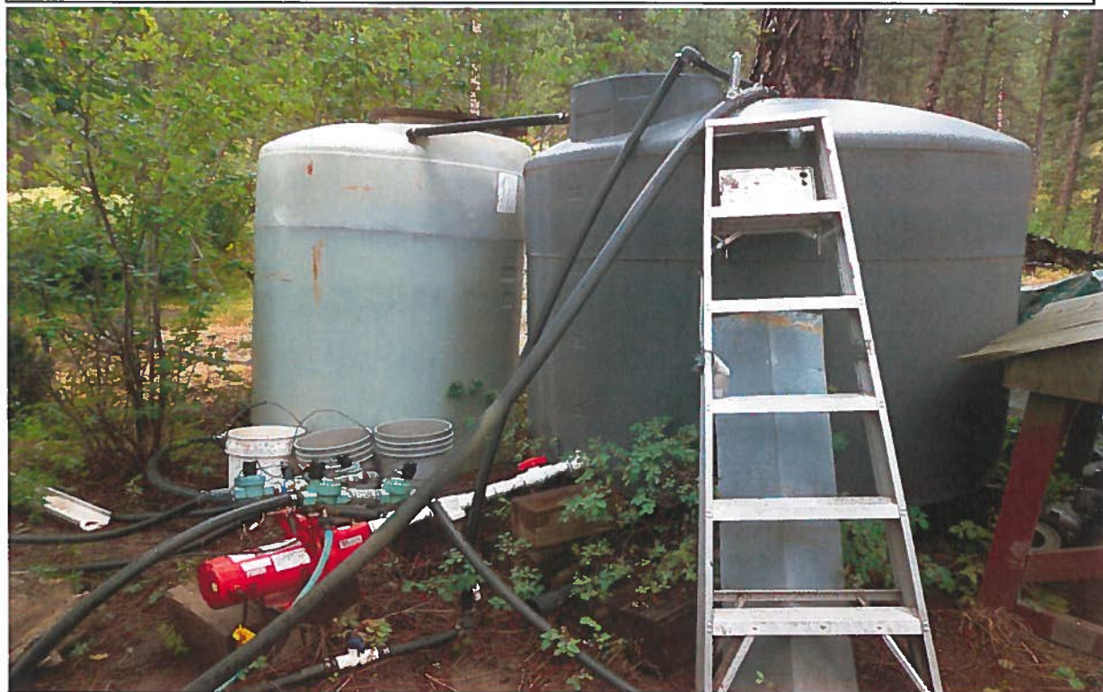
View northwesterly of a 500-gallon fiberglass storage tank and a 1,000-gallon fiberglass storage tank, which are designated for irrigation and fire protection. The 1 1/2" PVC discharge line is shown discharging through the top of the 1,000 gallon storage tank. Water levels in the storage tanks are manually operated. A 1 1/2-hp pump is connected to the 1 1/2" PVC discharge pipe from the 1,000-gallon fiberglass storage tank for irrigation and fire suppression. The solenoid valves shown are part of the properties irrigation system. The 1 1/2" PVC pipe connecting the two tanks is the fill line from the 1,000 gallon storage tank to the 500-gallon storage tank. The fire suppression system is comprised of sprinklers placed along the outer edge of a road which surrounds the home.
