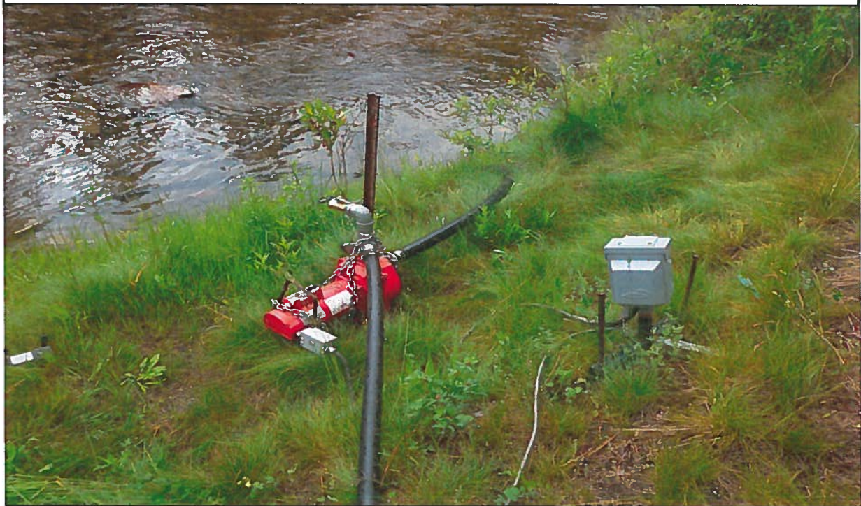
View southeasterly of the 2-hp Red Lion lawn and turf pump. The 2" PVC suction line is shown extending from the river to the pump. The pump discharges water through 1 1/2" PVC pipe to the right holder's property. The discharge pipe remains above ground to the right holder's property where the water is discharged into two fiberglass storage tanks.
