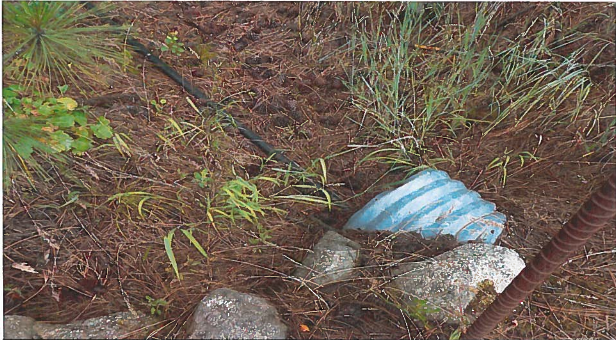
View of the 1 1/2" PVC discharge pipe exiting a culvert pipe crossing S. Middle Fork Road.
