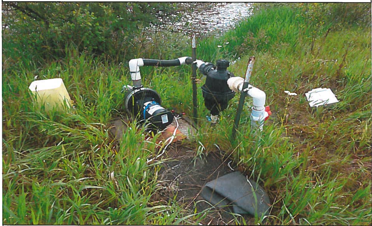
View easterly of the 2-hp centrifugal pump, 2" flexible hose suction line, and the 2" PVC discharge line on the west bank of the Middle Fork of the Payette River.
