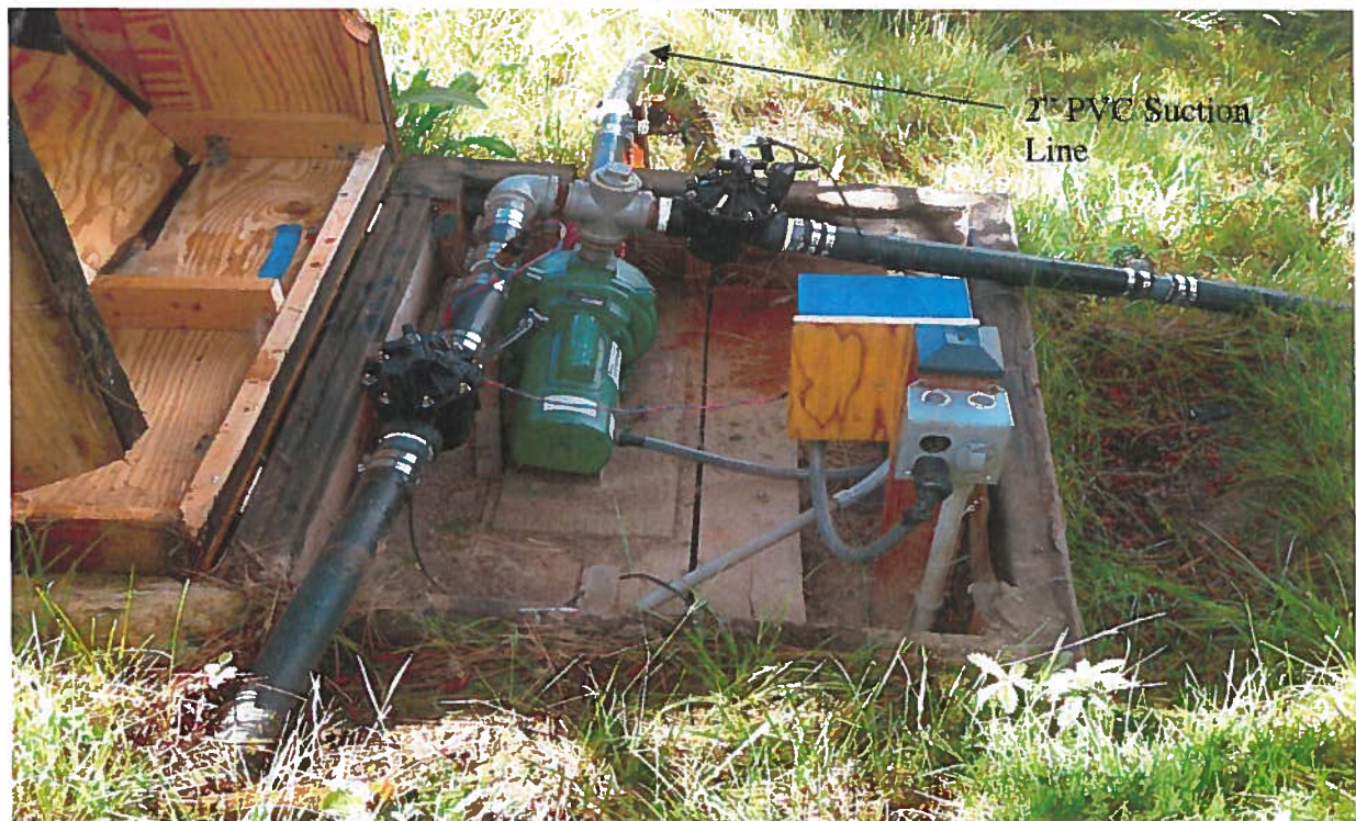
View westerly of the 2-hp centrifugal pump, 2" PVC suction line from the river, and two 2" PVC discharge lines to the right holder's pressurized irrigation system. The pump, solenoid valves, and junction box are located in a locked wooden enclosure.
